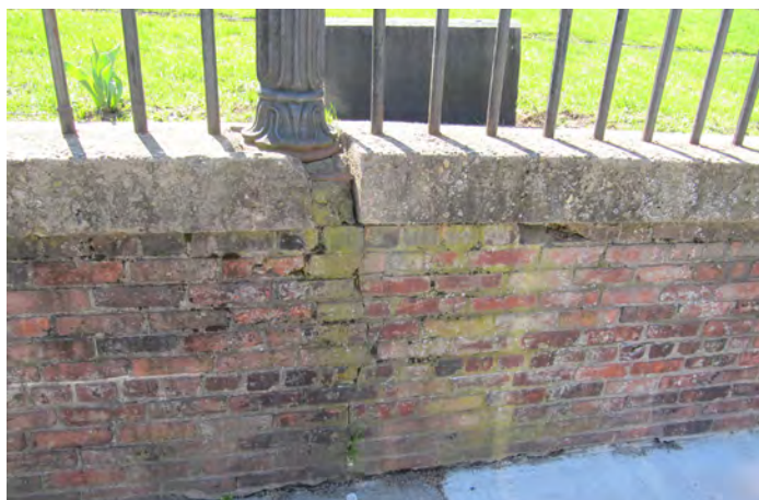
The concrete capstone was poured over the bottom of the fence post causing rusting and spalling.
