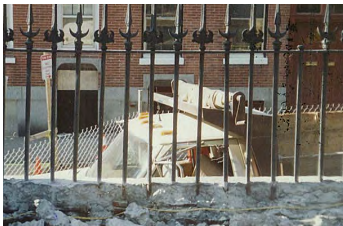
A photo from the 1992 Hull Street fence restoration shows the old concrete capstone partially removed. Notice the rusty picket ends.
