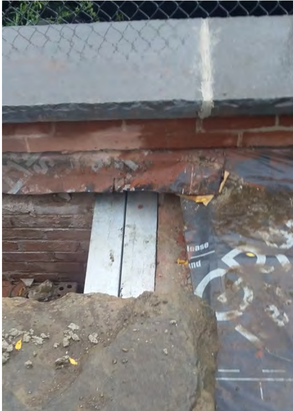
The new knee wall with bluestone cap is in the rear of the photo. The steel angle irons which support the gaps between the roof slabs are in the centre of the photo.
