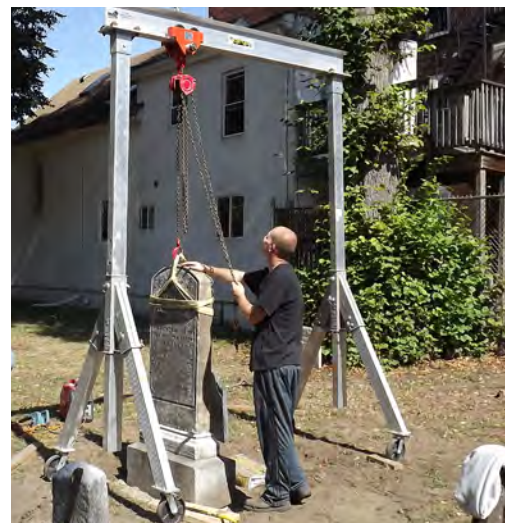
D.1: Conservators resetting a headstone which had fallen off its bases.
