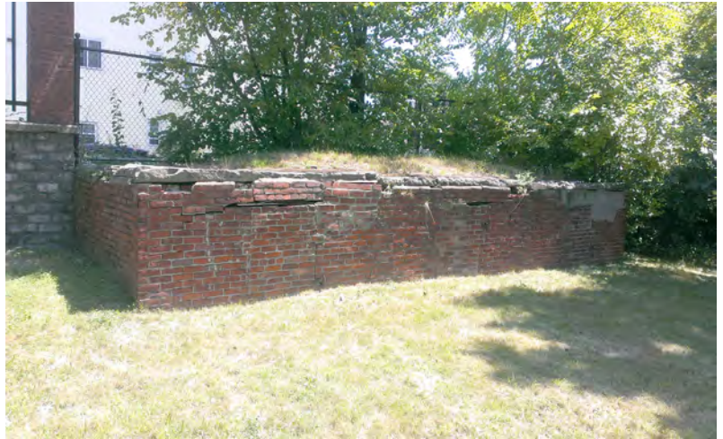
This is the east tomb structure before it was repaired. There are three individual tombs inside the structure. The doors have been bricked over. The trees behind the tombs ended up complicating the project greatly.
