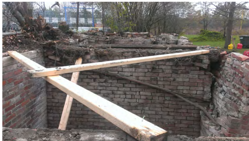
Inside the tomb once the roofs slabs have been removed. Some areas have missing mortar or bricks. Notice the the large root which has grown diagonally cross the tomb wall and into the brick on the lower front wall. Also notice the numerous small roots on top of the tomb wall which grew between the different layers of brick and compromised the structural stability of this wall.
