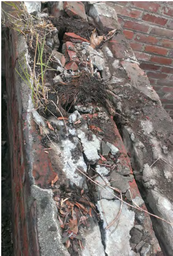
The different layers of brick in this sidewall had separated and were no longer structurally sound. A special structural grout was used to fill these cavities.
