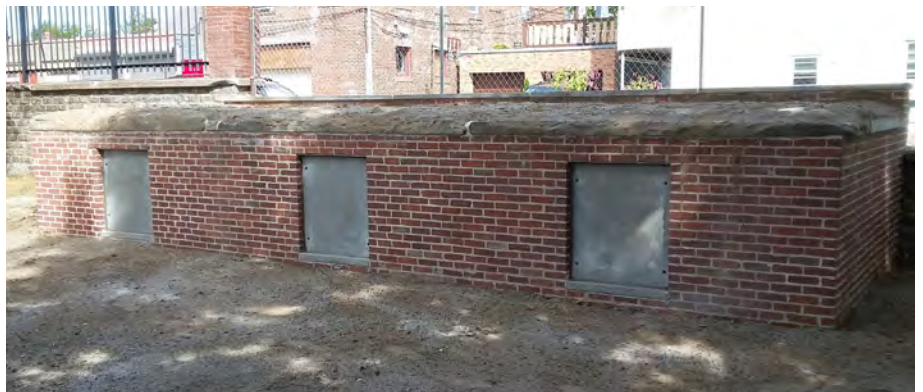
The tombs after the repair was completed (but before the grass seed grew in). The knee wall completely blends in with the original tomb wall.
