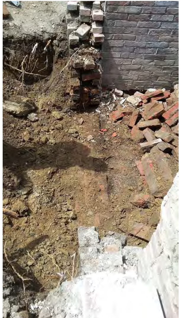
Upon closer inspection inside the tomb, it was discovered that the wall below the doorway on this tomb was unstable and had to be rebuilt.
