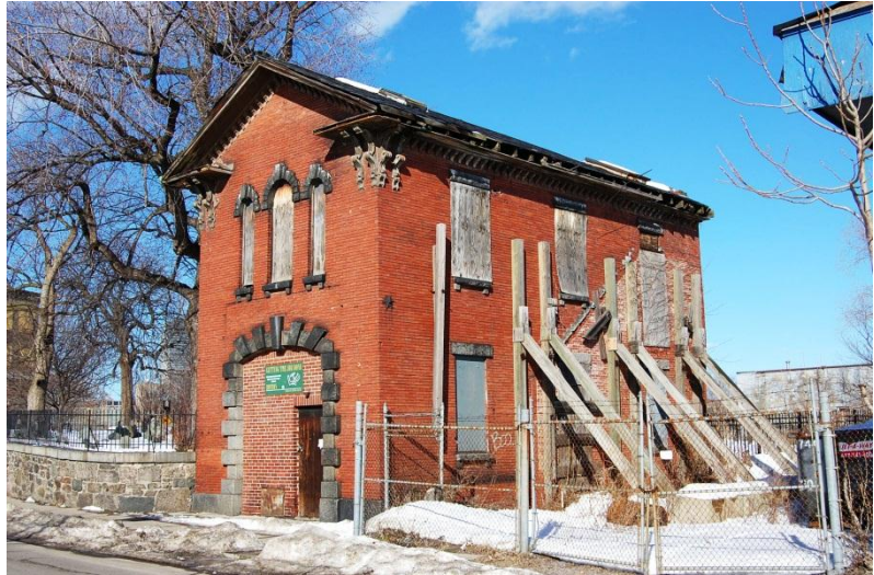
The old firehouse in 2009 before renovation. The reinforcements bracing the sides of the building were installed in the 1990s in order to keep the walls from falling down.
