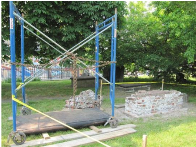
In order to rebuild the tomb base, the top slab had to be removed.
