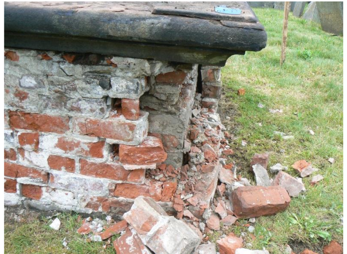
After the concrete parging was removed, the brick base was found to be in very poor condition.
