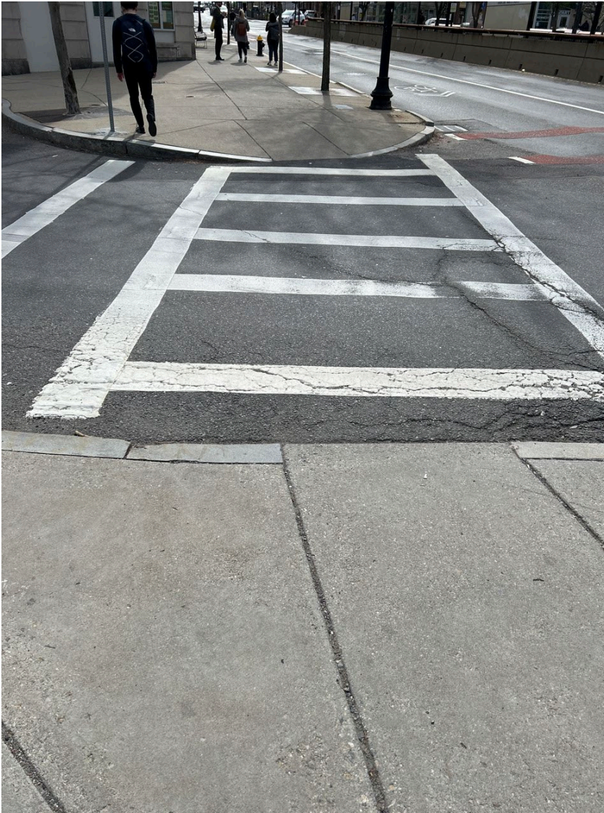
Figure 23 Crosswalk without Curb Ramps at Huntington Ave & St Alphonsus St
