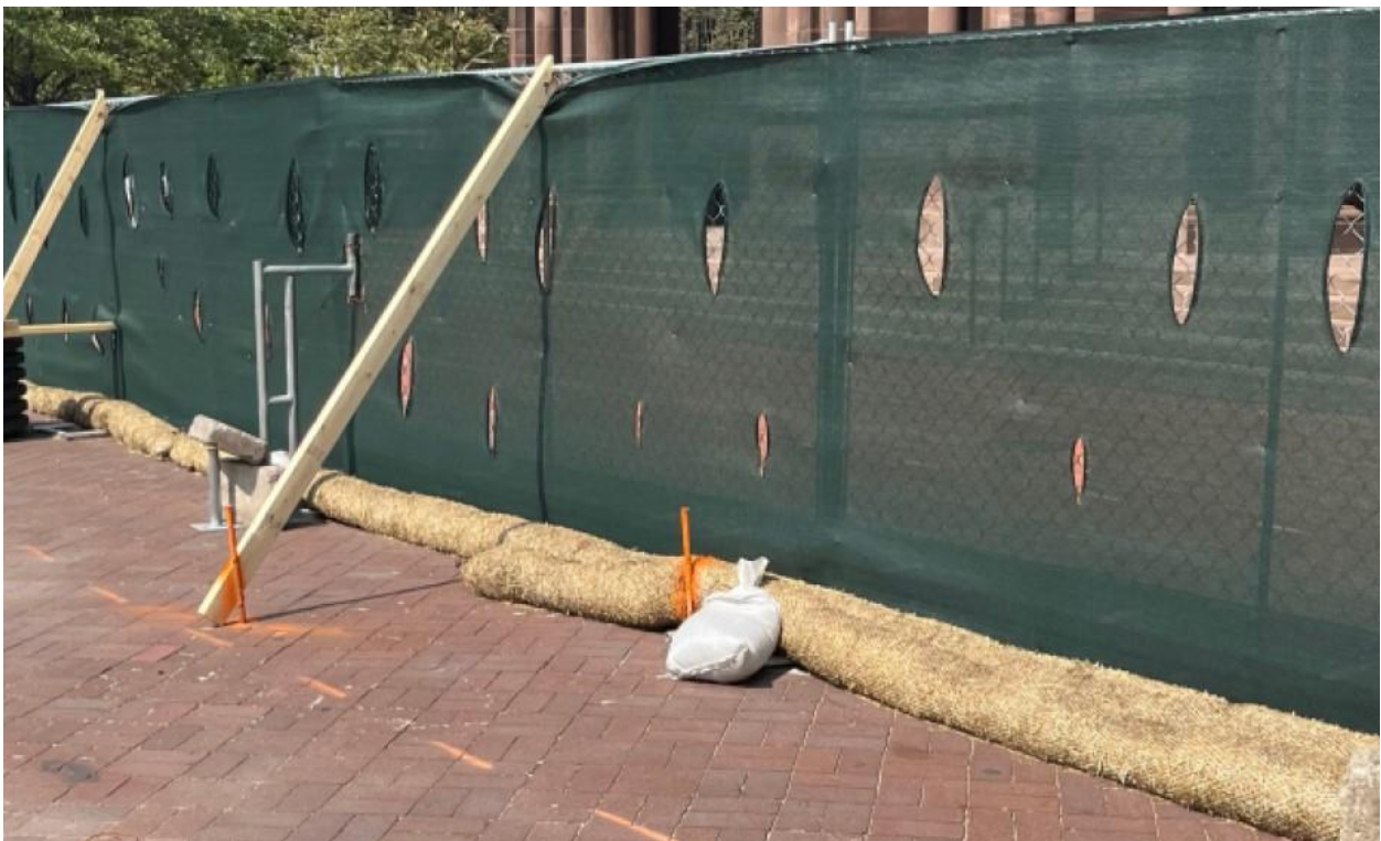
Screening has been installed on the fences to trap dust, and straw wattles prevent any silt-laden runoff from leaving the site.
