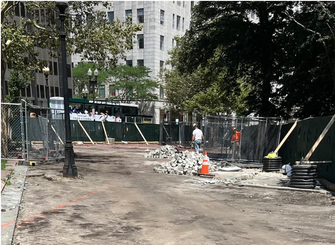
Pavement being removed: Granite blocks ready to go to the Maintenance yard, for future reuse.
