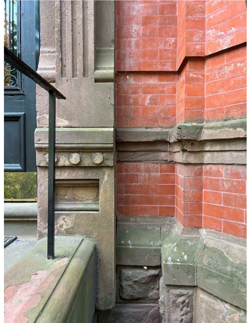
Damaged brownstone and efflorescence
