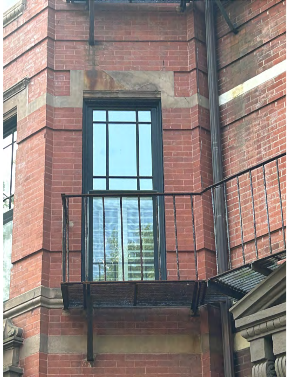
Third floor window with staining
