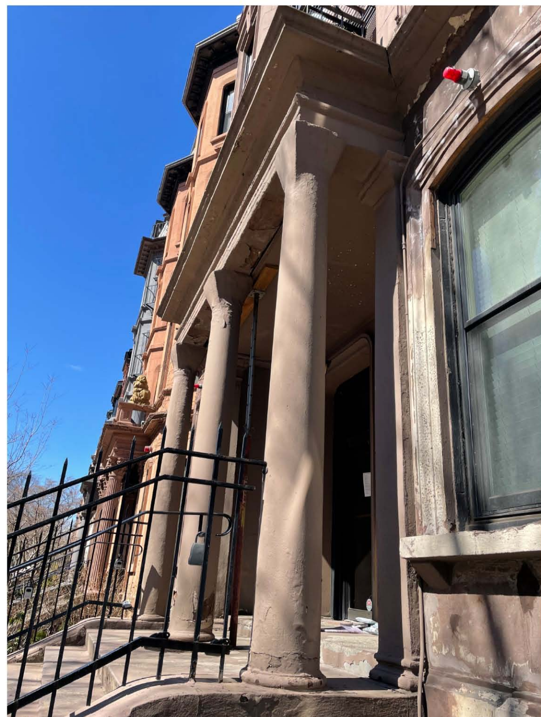
⑤ PHOTO OF DETERIORATED FRONT ENTRANCE PORTICO
