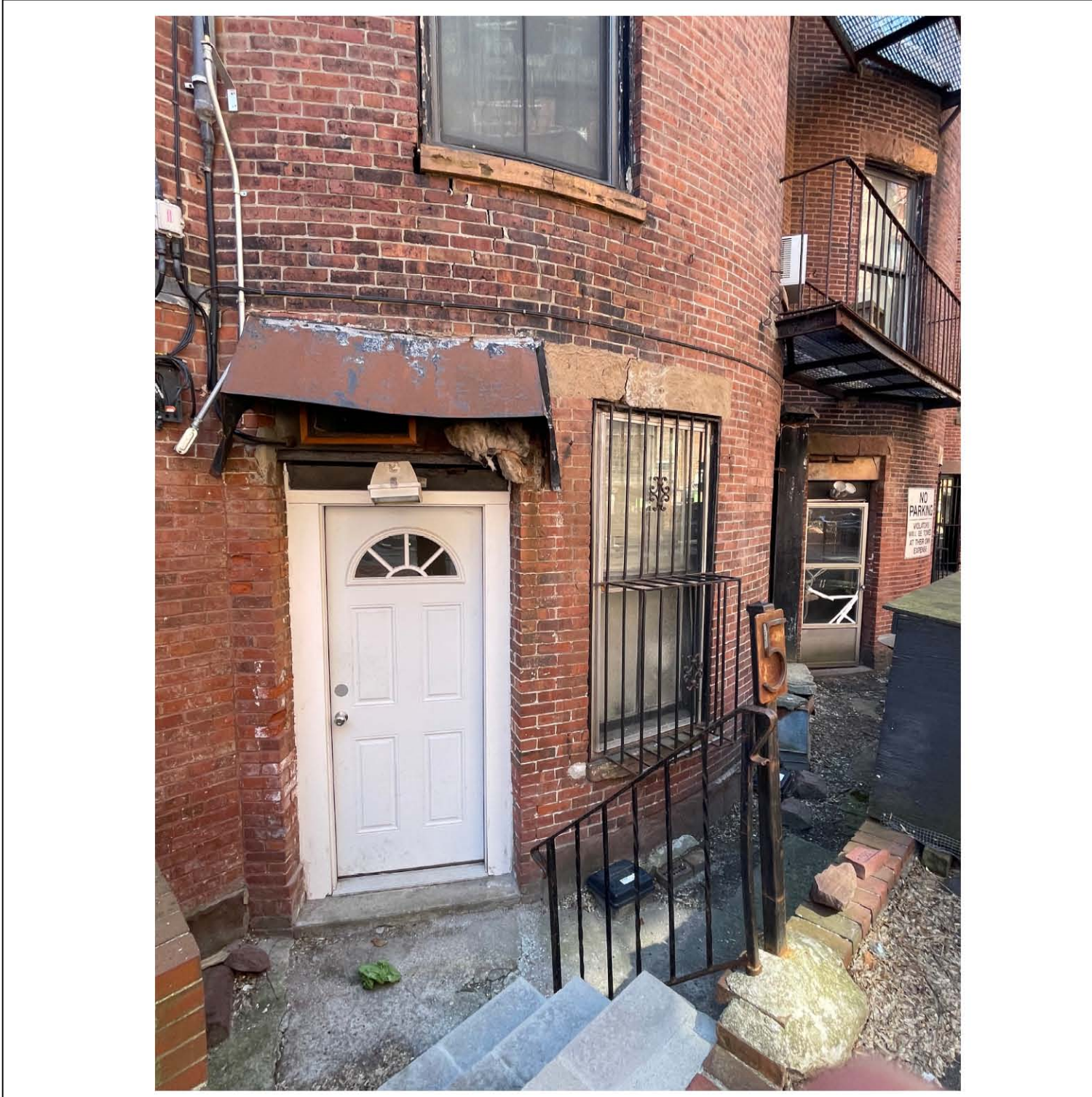
⑤ PHOTO OF NO. 9 INAPPROPRIATE REAR DOOR
