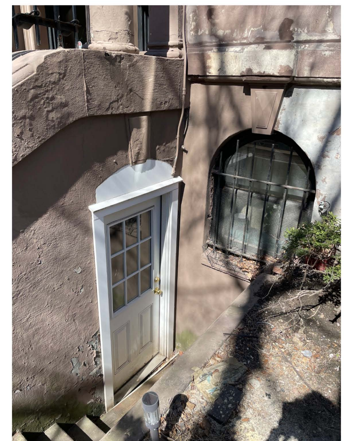
⑧ PHOTO OF INAPPROPRIATE NO. 9 LOWER DOOR
