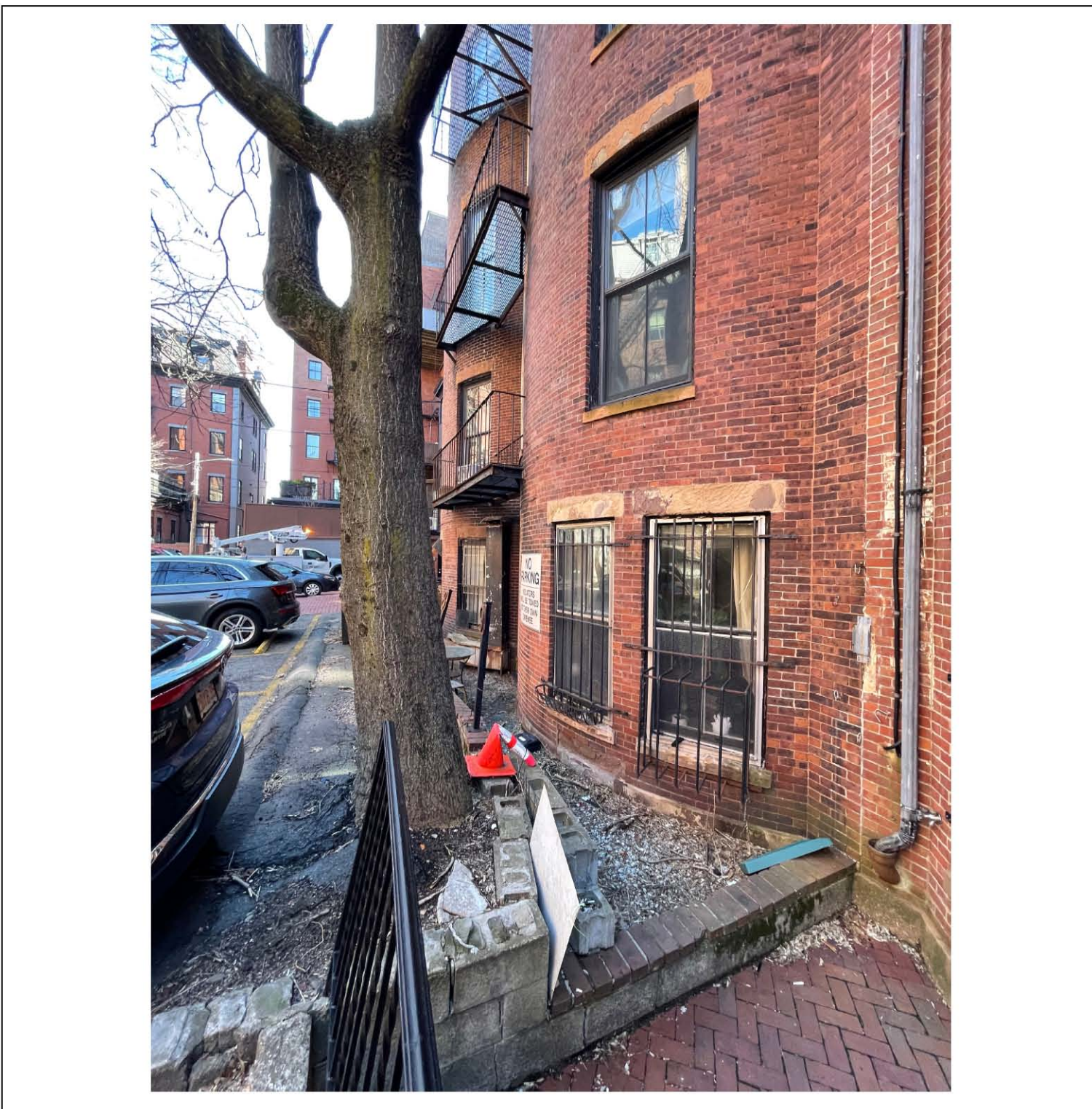
④ PHOTO OF DETERIORATED RETAINING WALL
