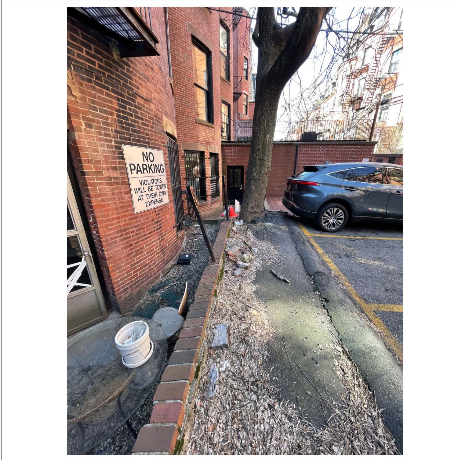
⑦ PHOTO OF DETERIORATED RETAINING WALL
