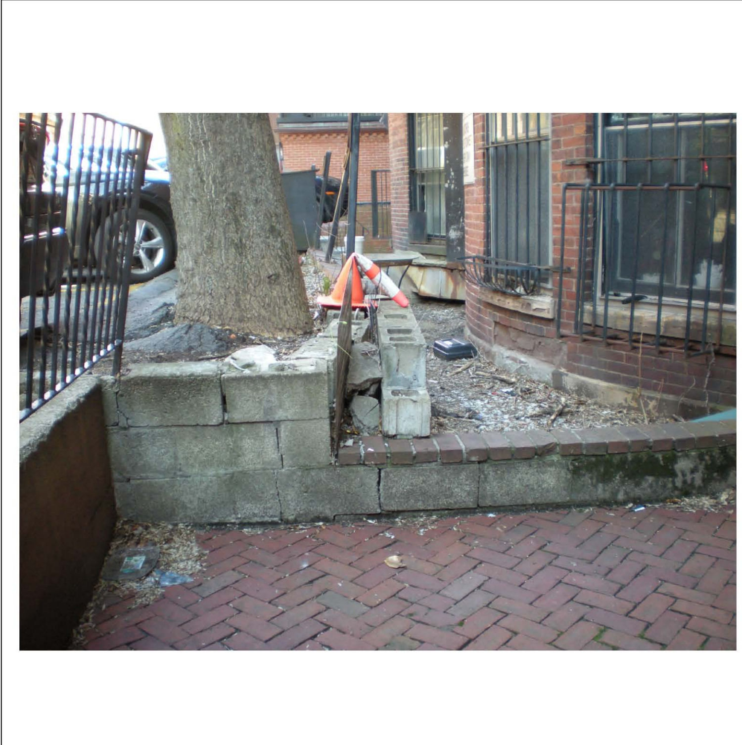
⑧ PHOTO OF DETERIORATED RETAINING WALL
