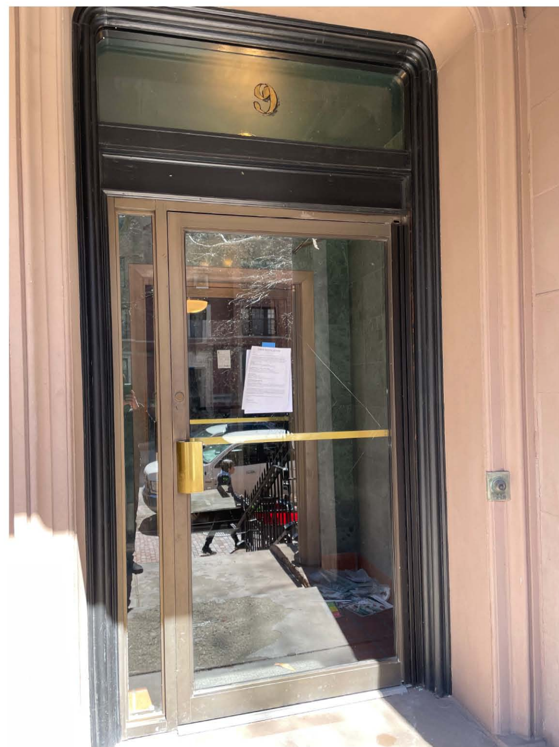
⑥ PHOTO OF INAPPROPRIATE METAL ENTRANCE DOOR
