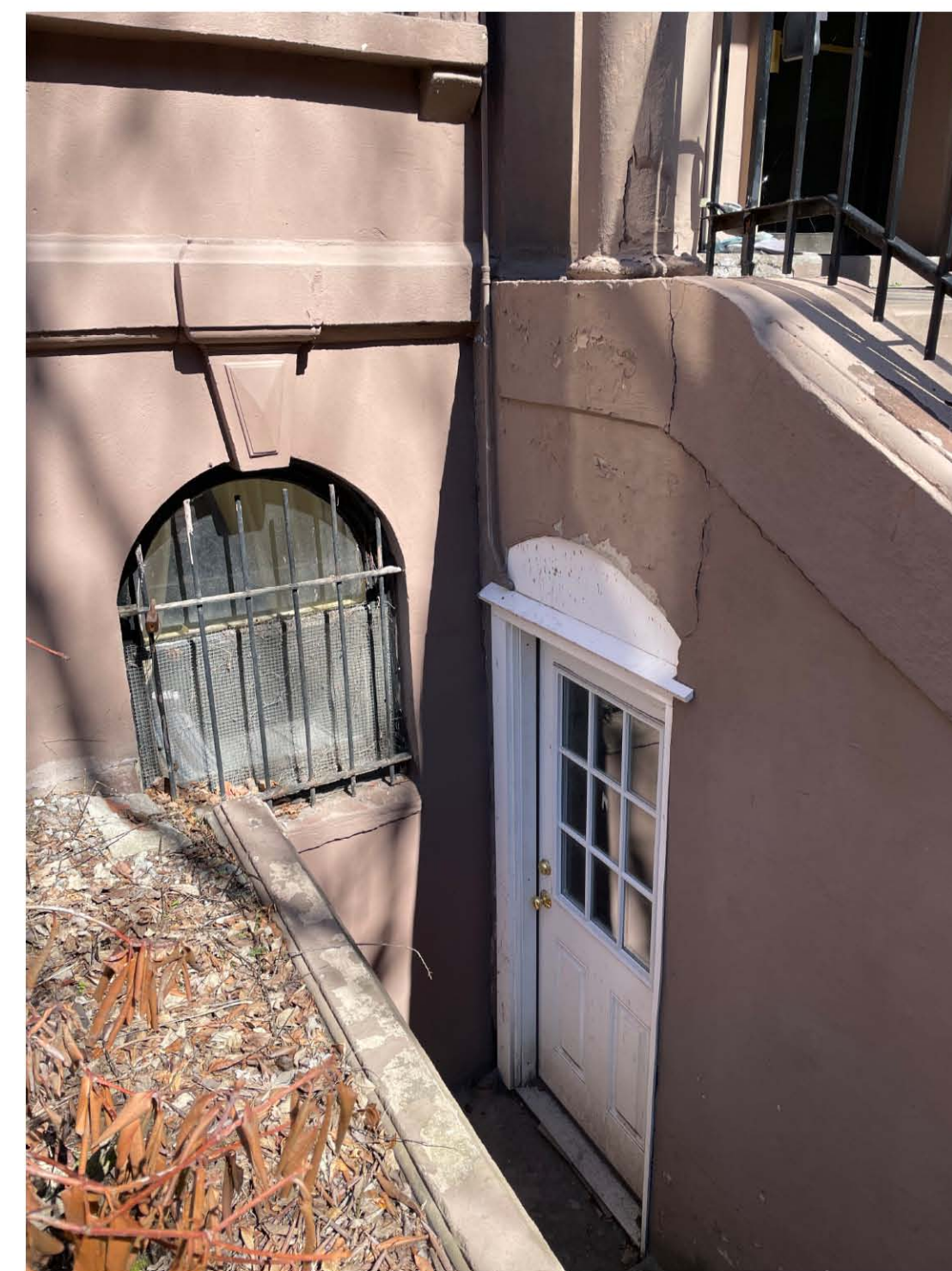
⑦ PHOTO OF INAPPROPRIATE NO. 11 LOWER DOOR
