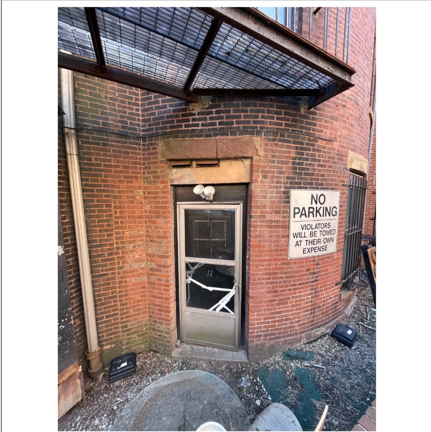
⑥ PHOTO OF NO. 11 DETERIORATED REAR HEADER
