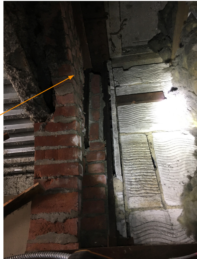
MISSING DECORATIVE STONE
