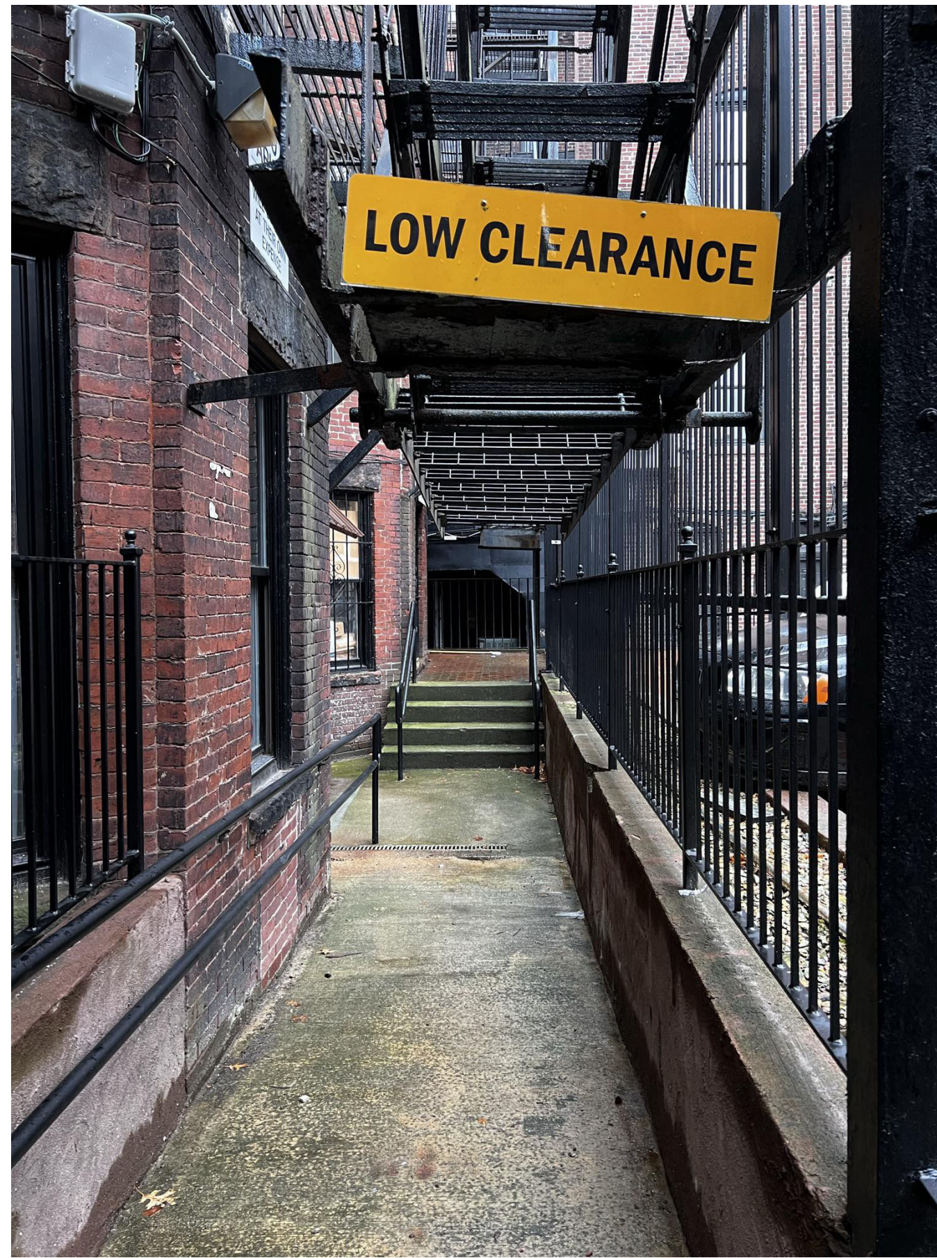
EXISTING RAMP AND WALKWAY TO BE REPLACED W/ CONCRETE PAVERS; WALLS TO BE PARGED AND PAINTED, SECOND HANDRAIL ADDED
