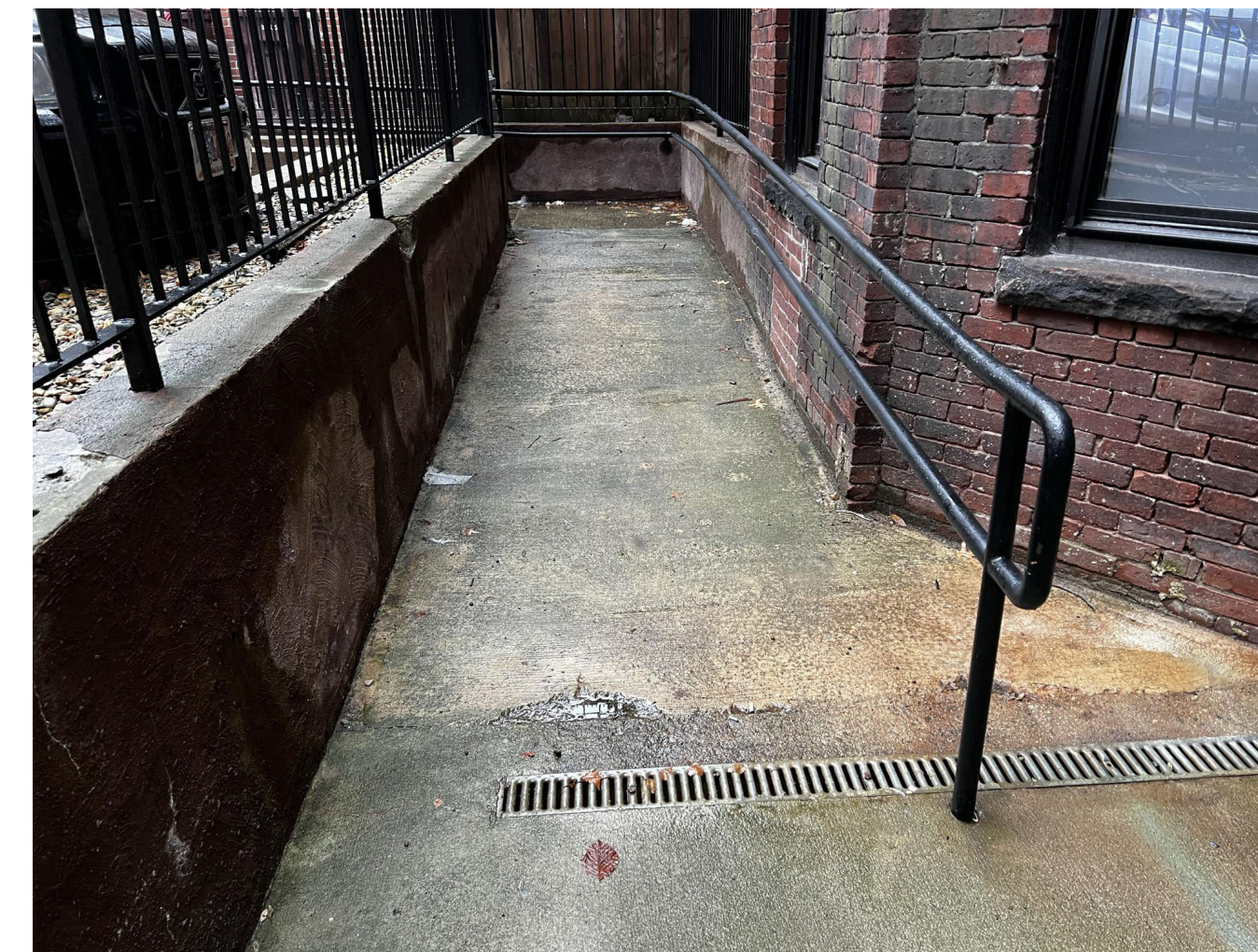
EXISTING RAMP AND WALKWAY TO BE REPLACED W/ CONCRETE PAVER, RAIL CUT BACK, SECOND HANDRAIL ADDED, WALLS TO BE PARGED AND PAINTED
