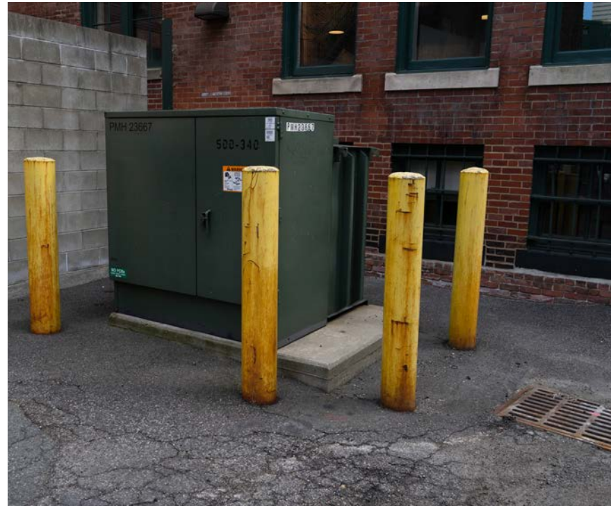
EXISTING EVERSOURCE TRANSFORMER
