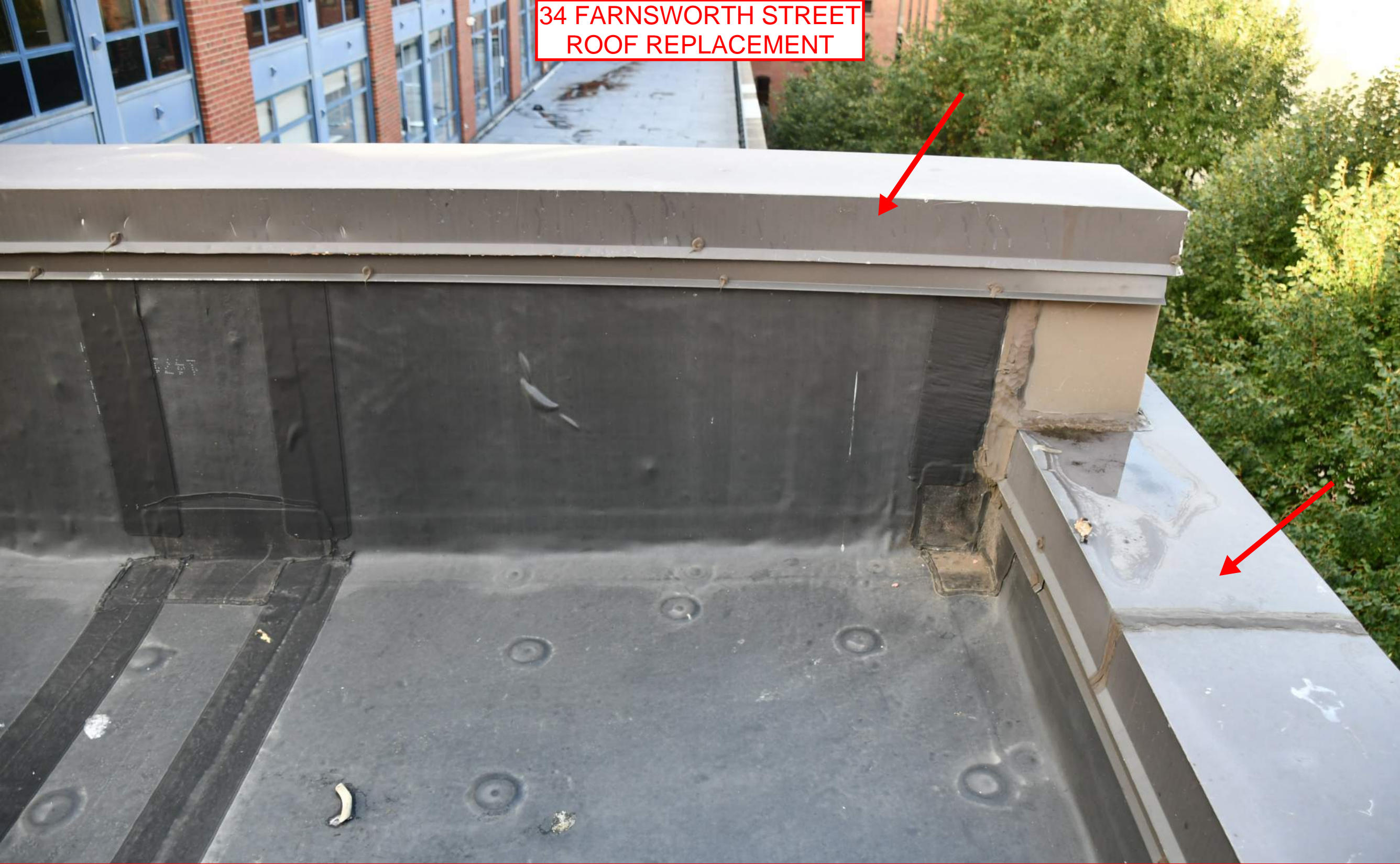
Close-up view of the existing aluminum parapet caps at the main roof, these will be replaced with copper caps. As you can see the EPDM membrane (black) runs under the caps and in order to replace the EPDM we need to remove the entire cap.
