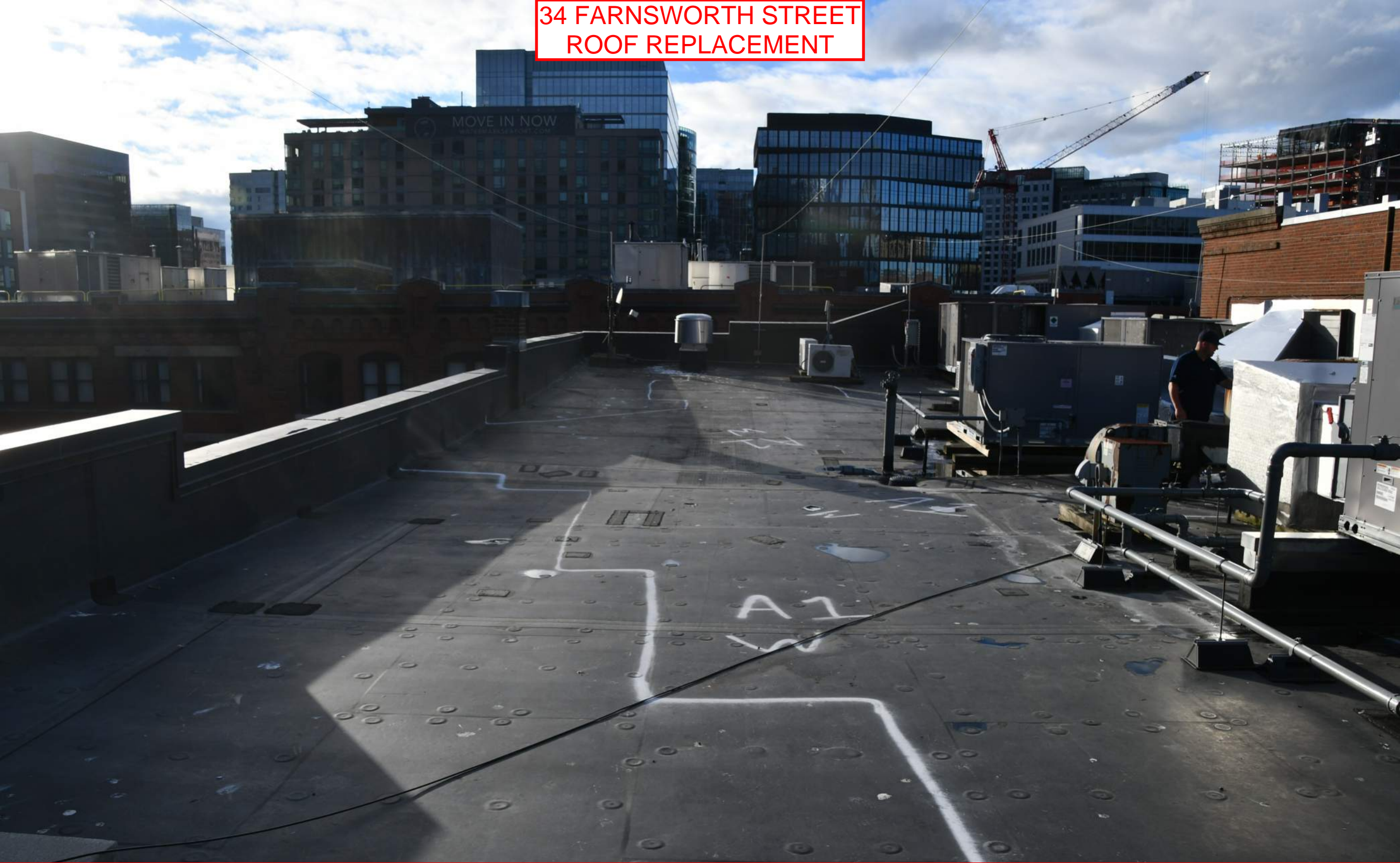
View of the existing EPDM roof at the main roof of the building, looking East.
