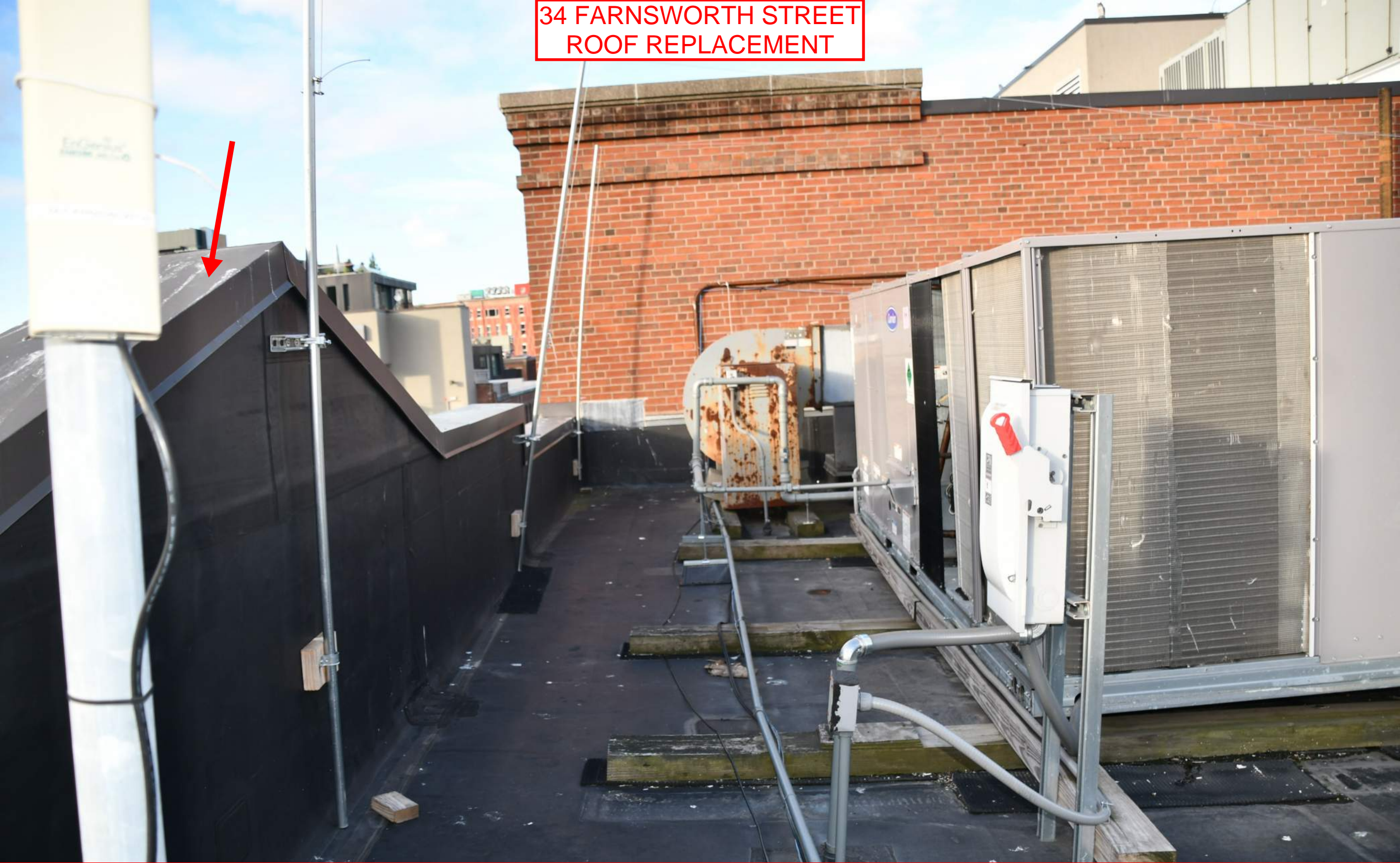
View of the East end of the main roof, looking South. Note the aluminum parapet caps that we would like to remove and replace with copper caps during the roof replacement.
