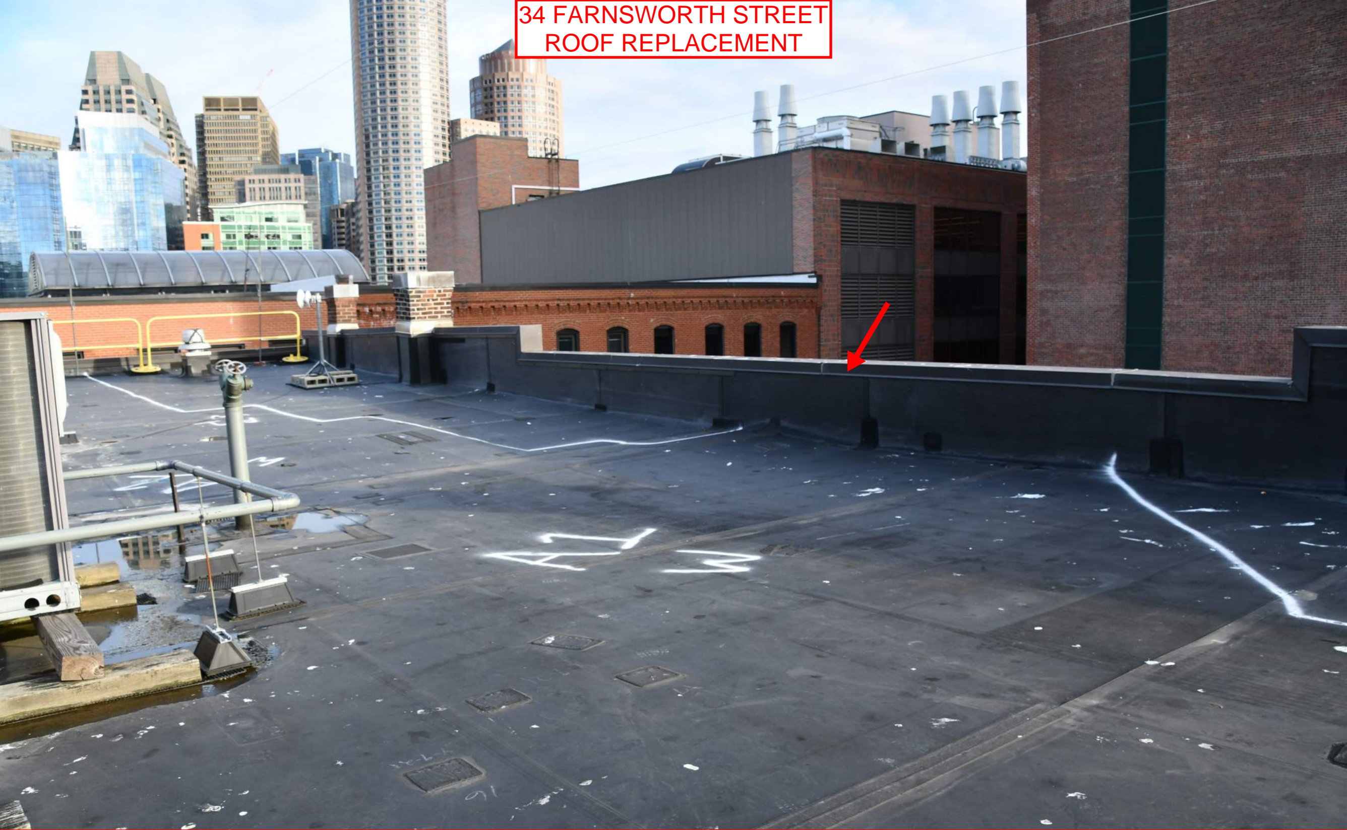
View of the existing EPDM roof at the main roof of the building, looking Northwest. Note the existing aluminum parapet caps which are to be replaced with copper caps. The EPDM goes up the wall and under the caps so the existing has to be removed in order to replace the entire roof system.
