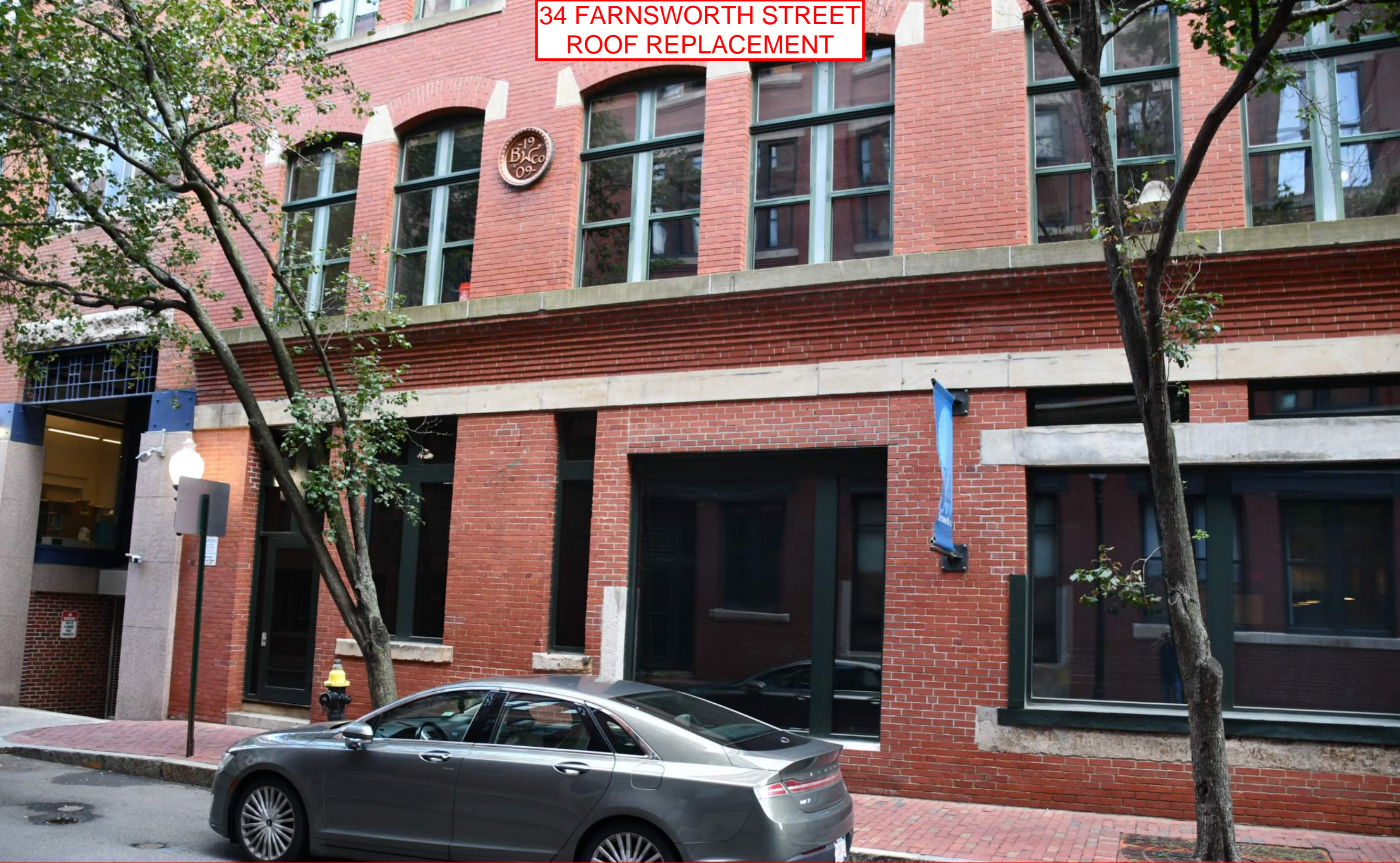
View of the first two floors of the East elevation of 34 Farnsworth along Farnsworth Street.
