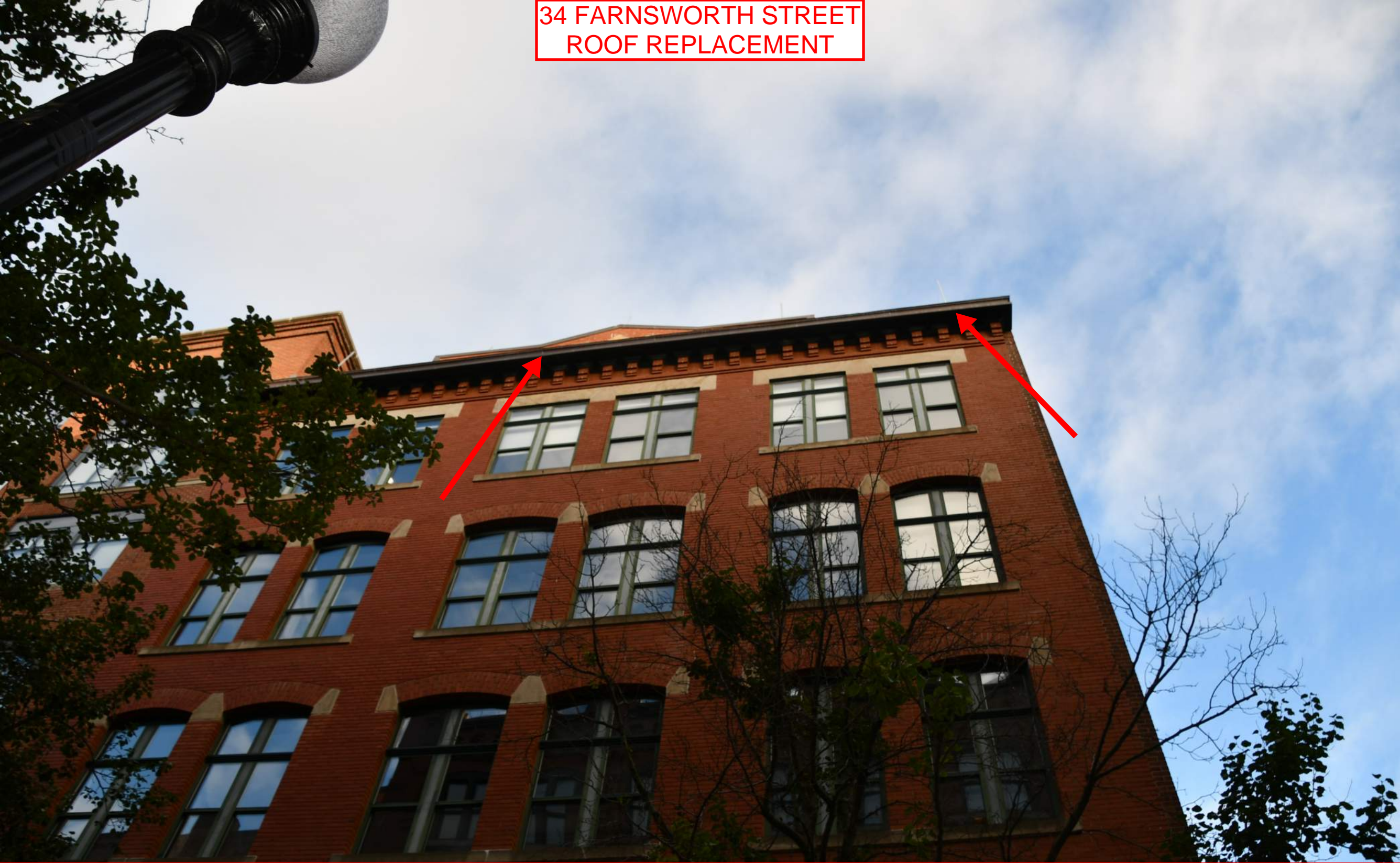
View of the upper floors of the East elevation of 34 Farnsworth along Farnsworth Street. Note the existing copper cornice below the roof edge. See the next photograph for a close-up view of this copper cornice, which is to remain.
