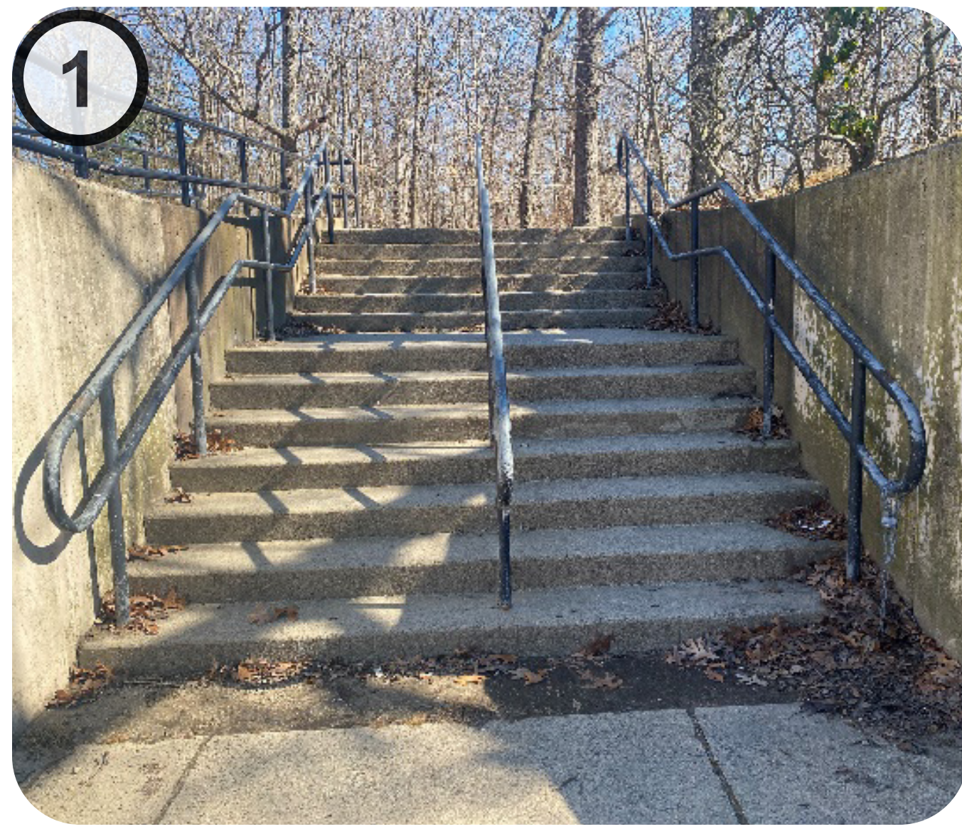
1 CONCRETE STAIRS WITH HANDRAILS IN FAIR CONDITION @ DORCHESTER AVE.
