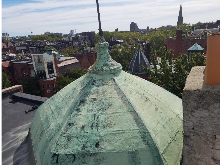
Photo 5: This photo shows existing coating and repairs to dome roof utilizing asphalt cement.
