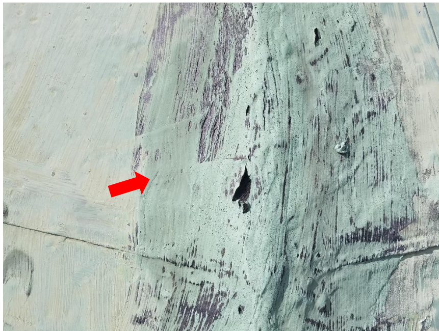
Photo 6: Photo shows close-up of incompatible asphalt repair and existing paint/coating on dome roof.
