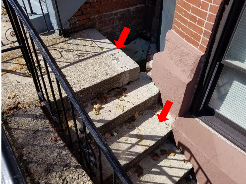
Photo 3: Replace cracked/deteriorated concrete steps leading to low level unit.
