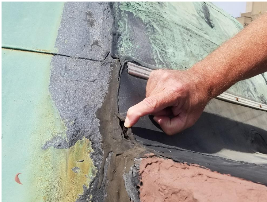
Photo 8: Improper flashing installation and repair, at copper dome roof flashing.
