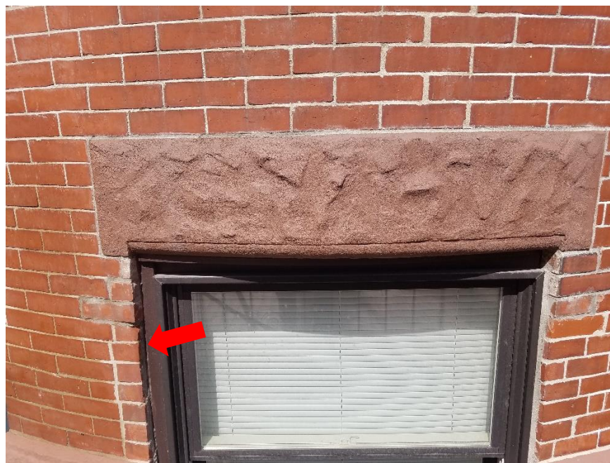
Photo 2: Seal open joint between brick veneer and window frame with approved bronze colored sealant.
