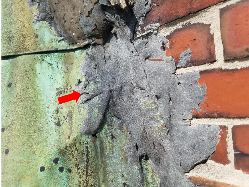
Photo 7: incompatible repair material (asphalt cement) on copper dome and flashings.
