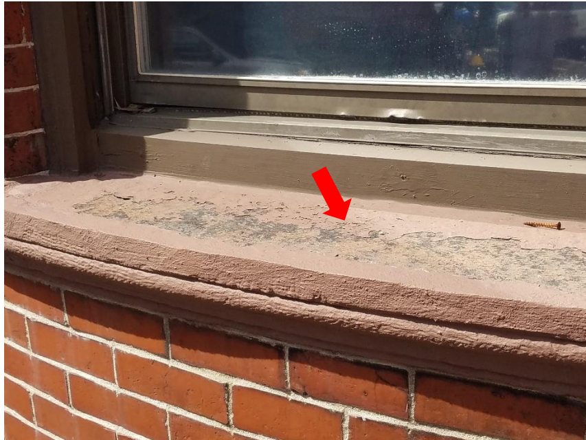
Photo 1: Deterioration of existing paint on concrete band, recommend repainting with compatible material.
