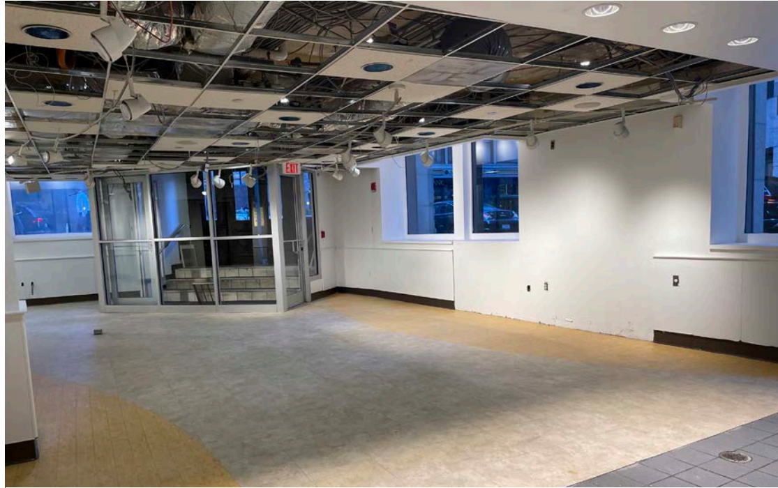
INTERIOR VIEW OF WINDOWS (NOTE THE SMALL TRANSOM WINDOWS ARE ABOVE THE CEILING PLANE)
