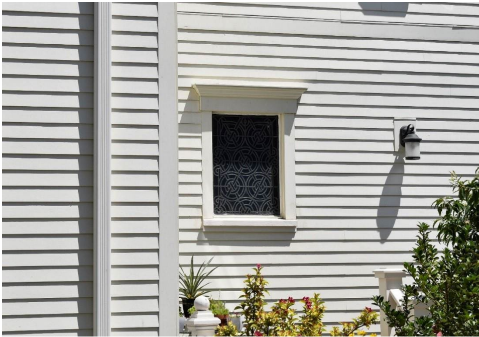
Figure 18. Detail of leaded glass window on the south elevation of the rectory, facing north. Taken June 20, 2022.
