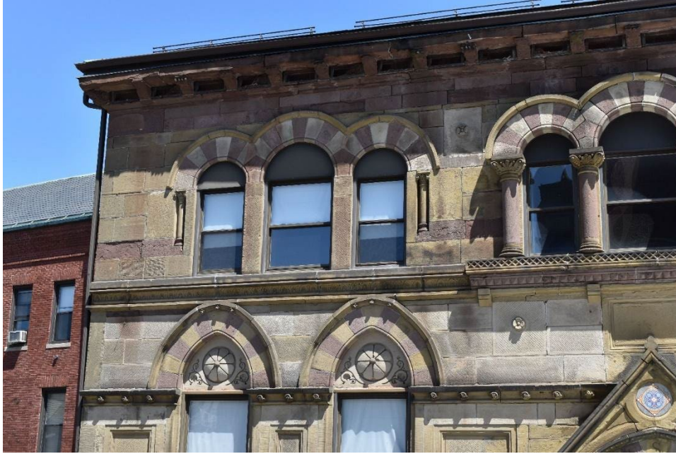
Figure 33. Detail of decorative trim on the south (rear) elevation of the Cheverus School, facing north. Taken June 20, 2022.
