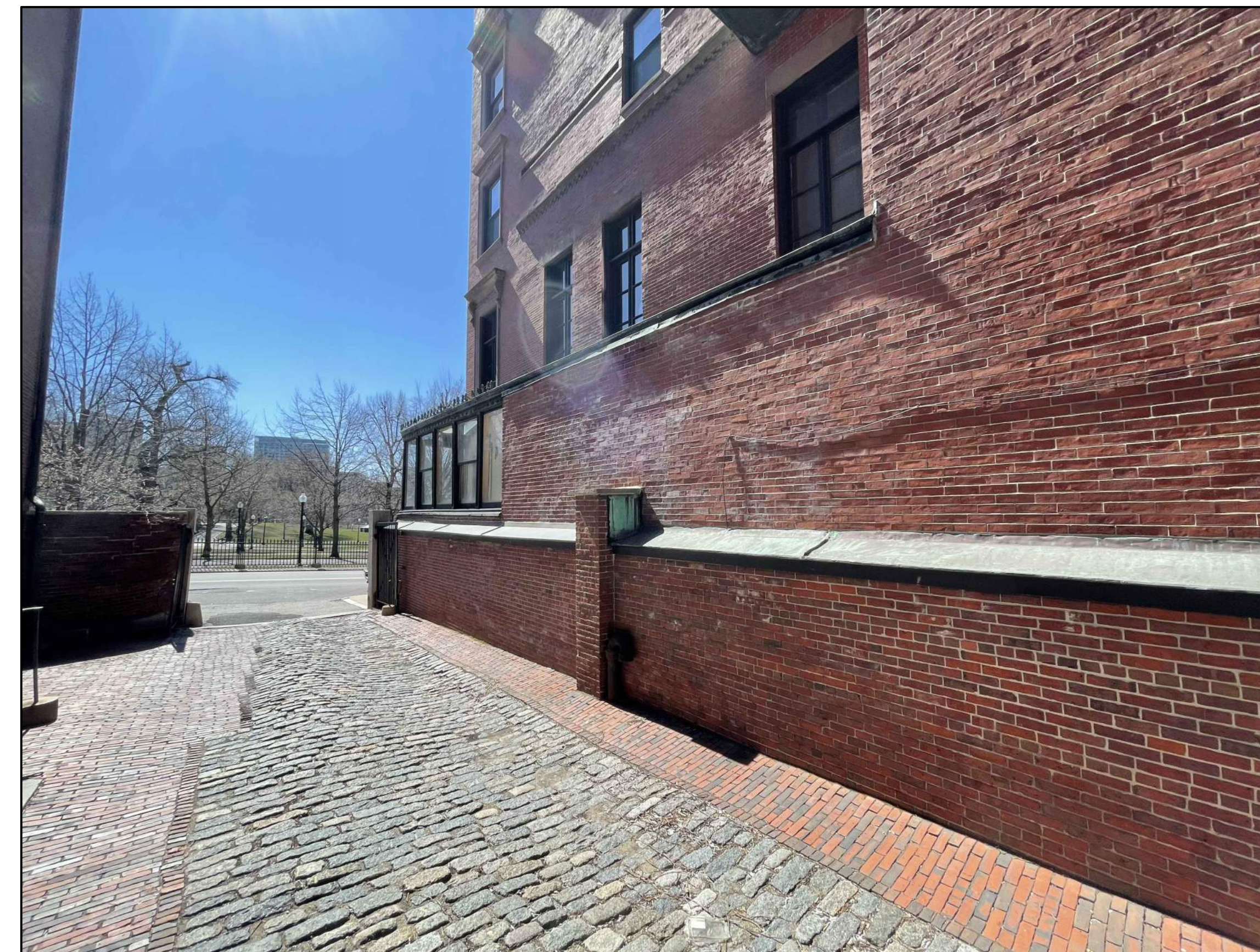
EFFLORESCENCE AND DISPLACED BRICK MASONRY
