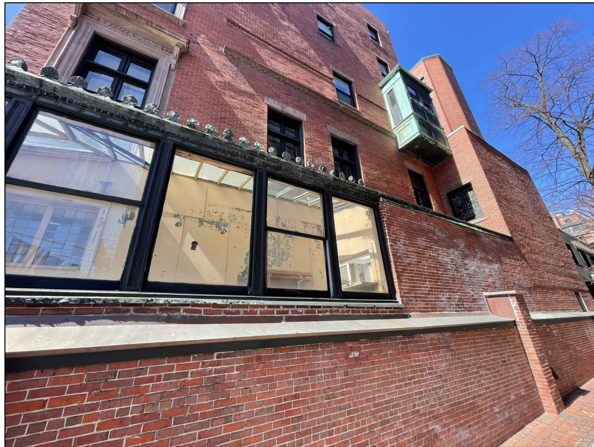
EFFLORESCENCE AND DISPLACED BRICK MASONRY
