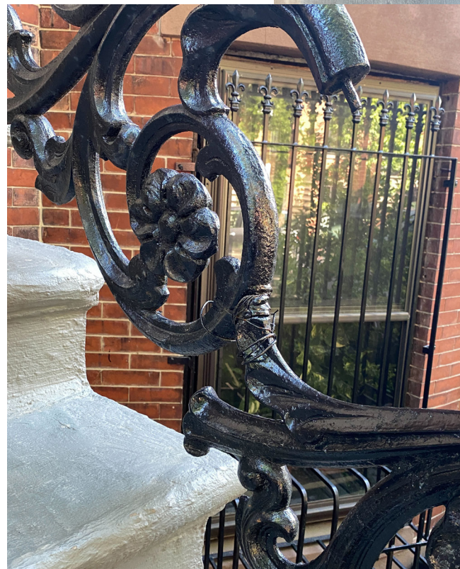
Damage on existing front railings
