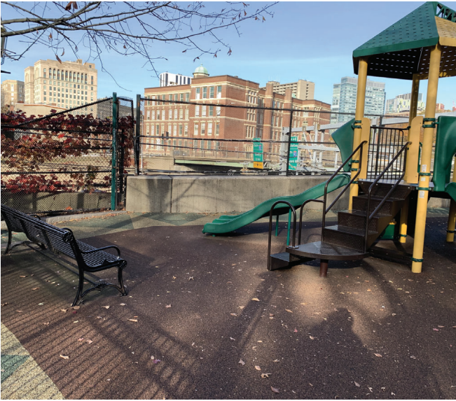
Damaged existing fence on concrete wall to be repaired/replaced to match existing.
