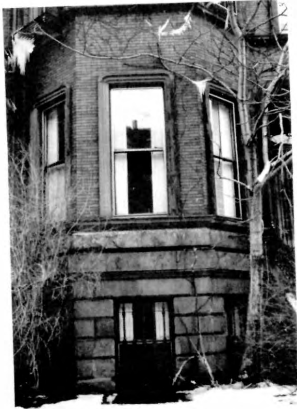
58 Windows of 4 Marlborough Street, 1864. A simplified Academic design in brick encases openings with plain brownstone architraves and omits the usual component of Classical details.
