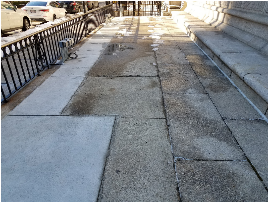
JJ: TERRACE BY CORNER OF FRANKLIN ST AND PEARL ST; NEW POURED CONCRETE ON LEFT, EXISTING POURED CONCRETE AND GRANITE PAVERS ON RIGHT
