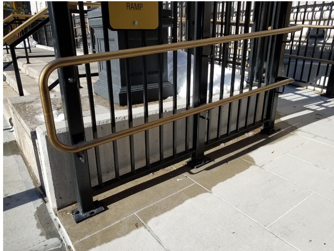
E: CONCRETE KNEE WALL FROM LOWER PORTION OF RAMP
