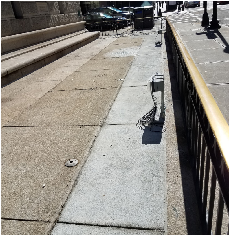
LL: TERRACE LOOKING TOWARD FRANKLIN ST; NEW POURED CONCRETE ALONG FENCE WITH ELECTRICAL/AV OUTLETS
