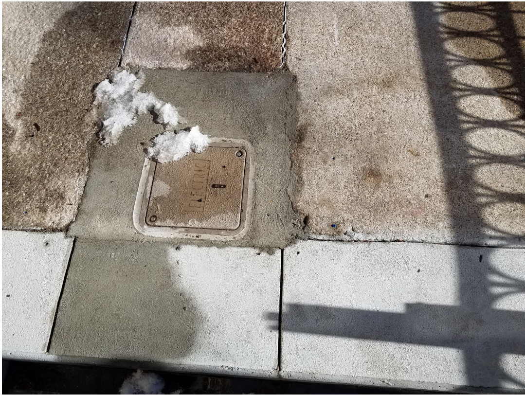
KK: NEW ELECTRICAL ACCESS PANEL
