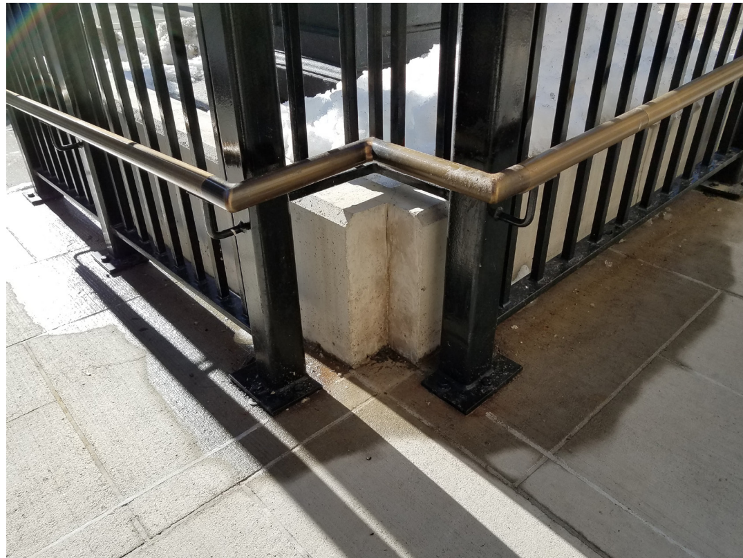
D: ADA/521 CMR REQUIRED NOTCH AT INNER CORNER OF INTERMEDIATE RAMP LANDING THE FED ACCESSIBLE RAMP
