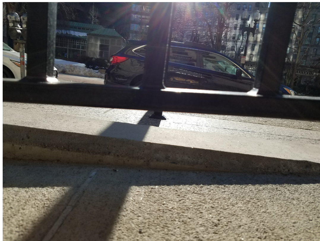
O: RAMP TO TOP LANDING TRANSITION THE FED ACCESSIBLE RAMP
