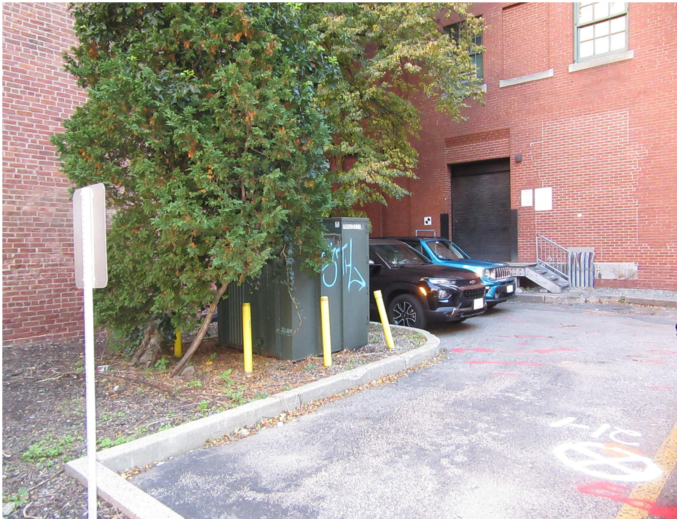
PHOTO 6 - 11 SLEEPER STREET TRANSFORMER - VIEW NORTHEAST
