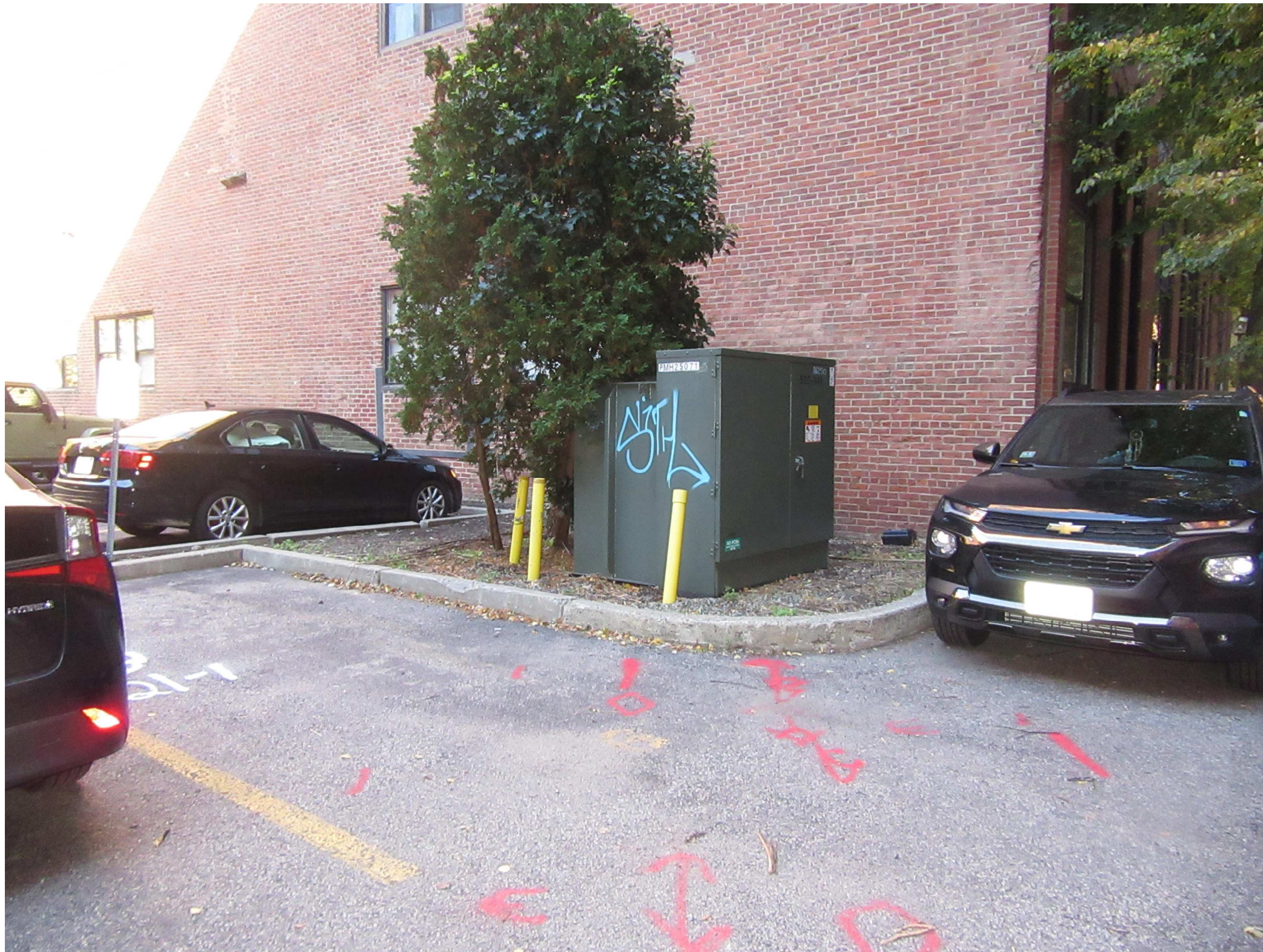
PHOTO 5 - 11 SLEEPER STREET TRANSFORMER - VIEW NORTHWEST
