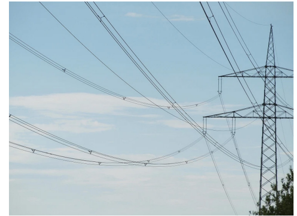
High voltage power lines power lines sagging in the heat
