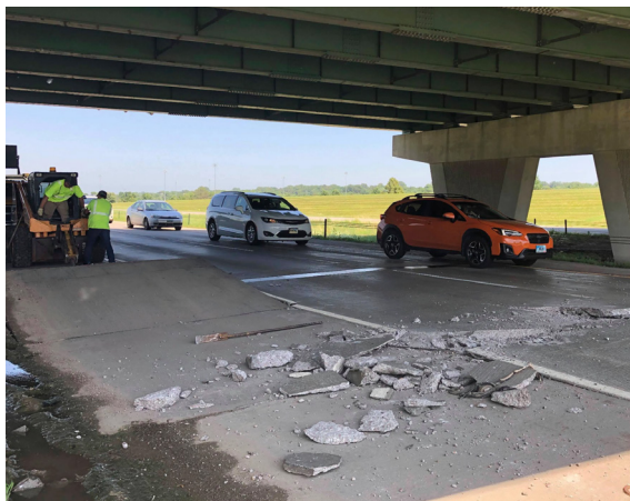
Roads buckling in extreme heat
