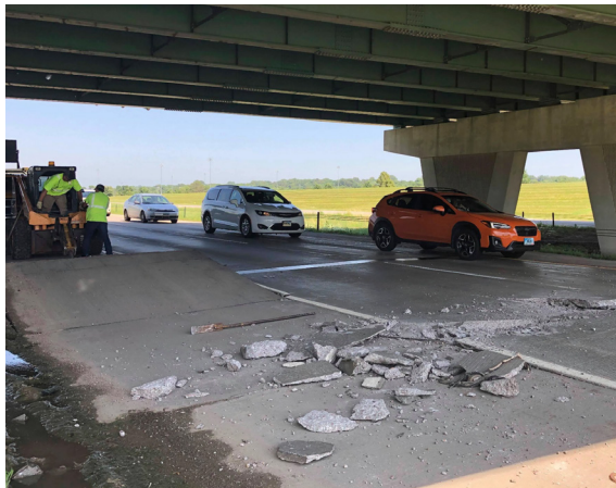
Roads buckling in extreme heat
