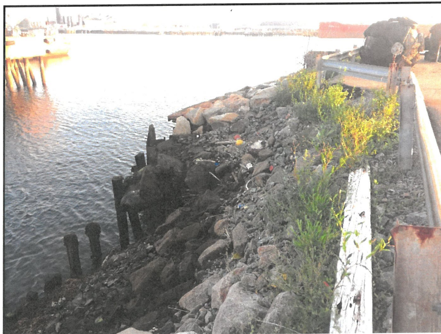
Typical Condition of Stone Revetment at Northern End of Western Stone Revetment
