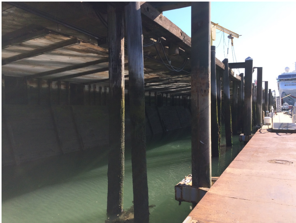
Photograph No.: 6 Thompson Island float and piles. View looking northeast toward EDIC Pier.
