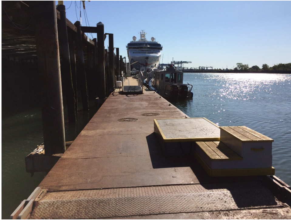
Photograph No.: 5 Thompson Island float and piles. View looking east in Reserved Channel.
