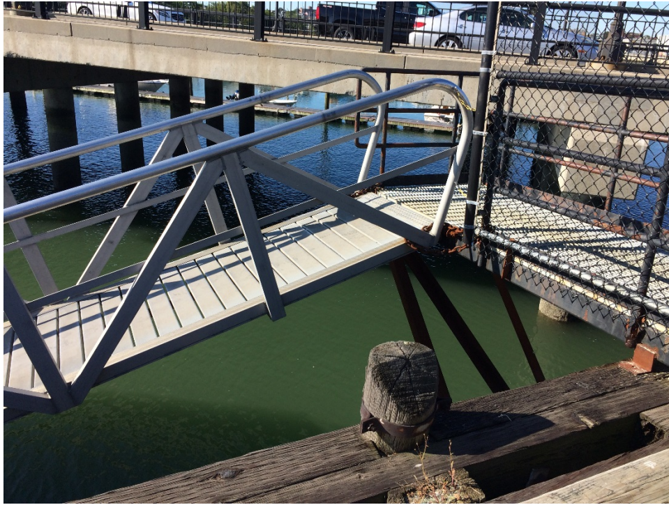
Photograph No.: 3 Thompson Island access pier and ramp connection looking southwest toward Summer Street.
