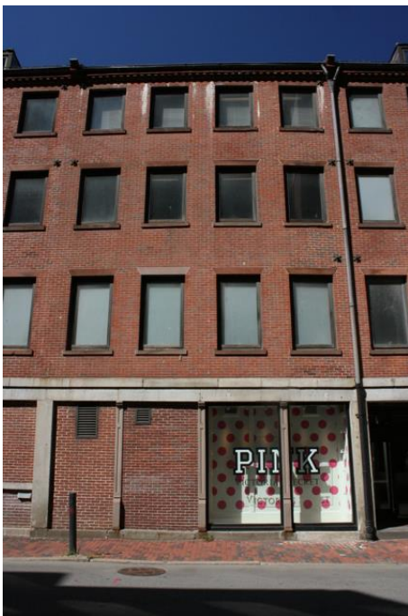
Figure 17. Back (south) elevation: Typical building unit with atypical cast iron pilasters at storefront.
