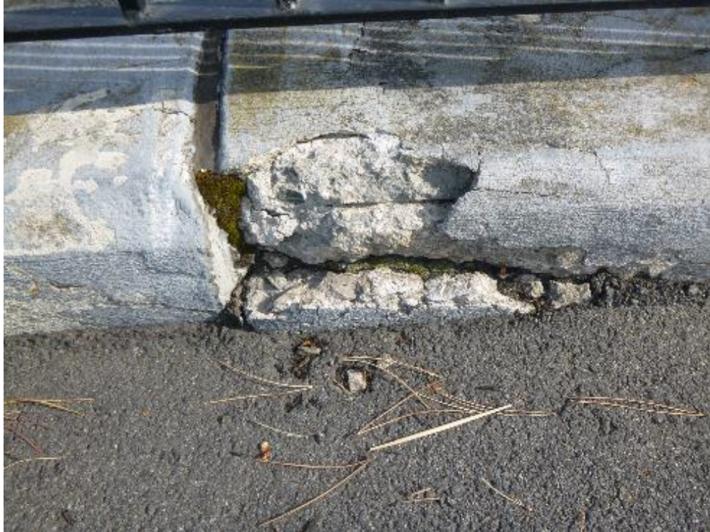
Photo 5: Typical concrete defect on the sheet pile cap.
