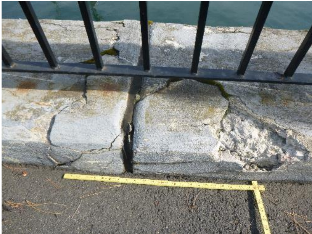
Photo 4: Typical concrete defect on the sheet pile cap.
