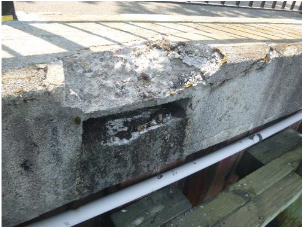
Photo 6: Typical concrete defect on the sheet pile cap.
