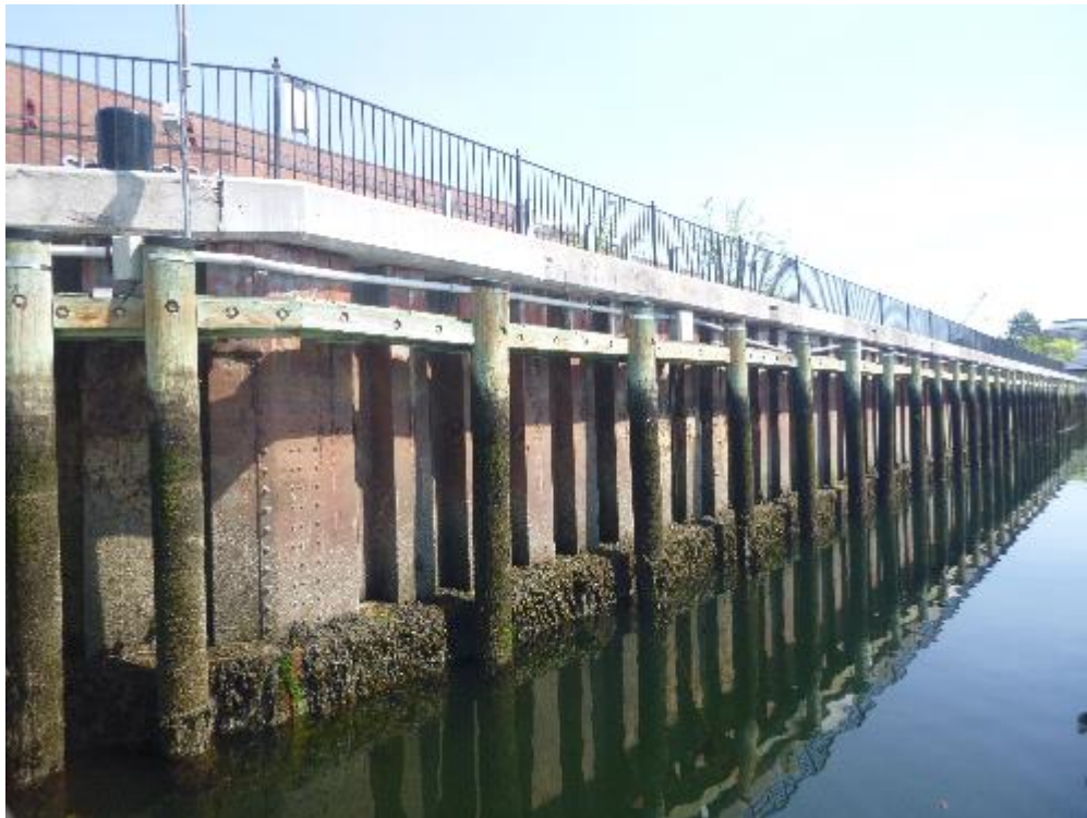
Photo 2: Overall view of the sheet pile bulkhead with concrete pile cap and handrails on top.
