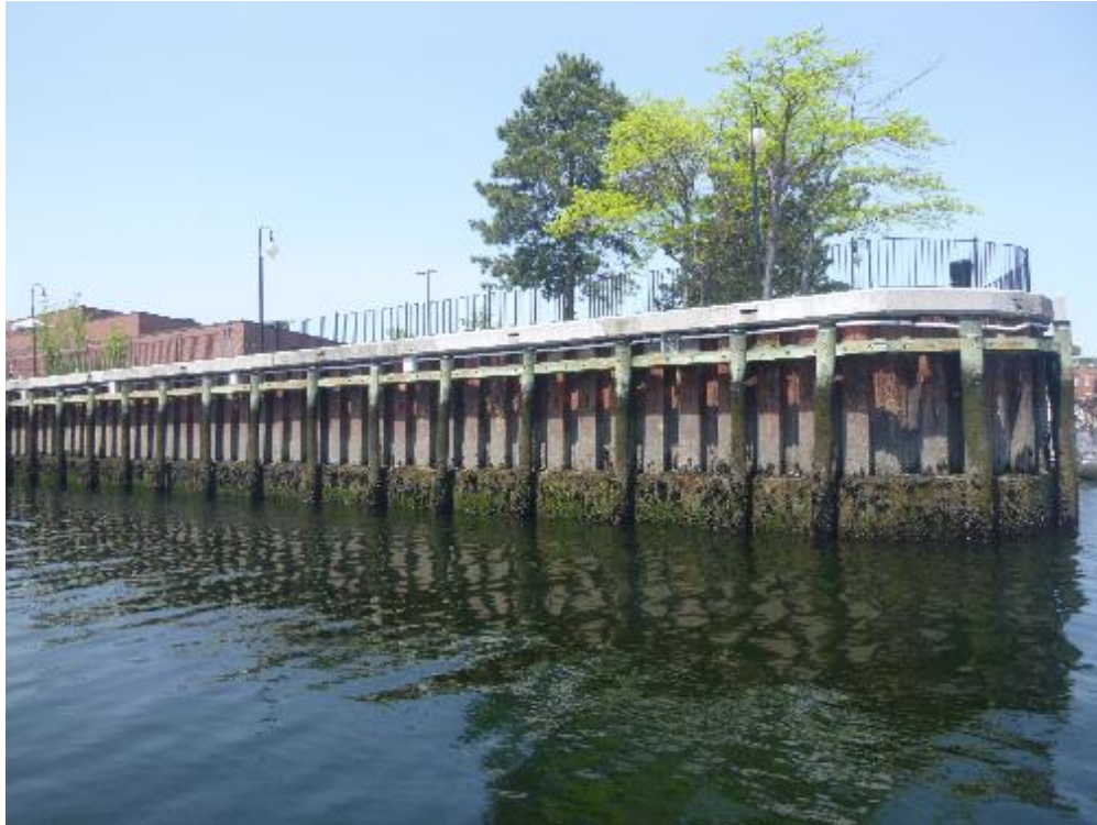
Photo 1: Overall view of the sheet pile bulkhead with concrete pile cap and handrails on top.
