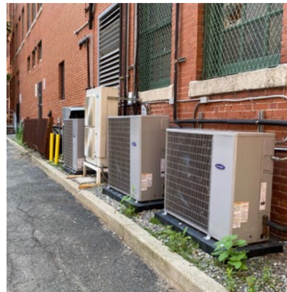
Existing Mechanical EQ
