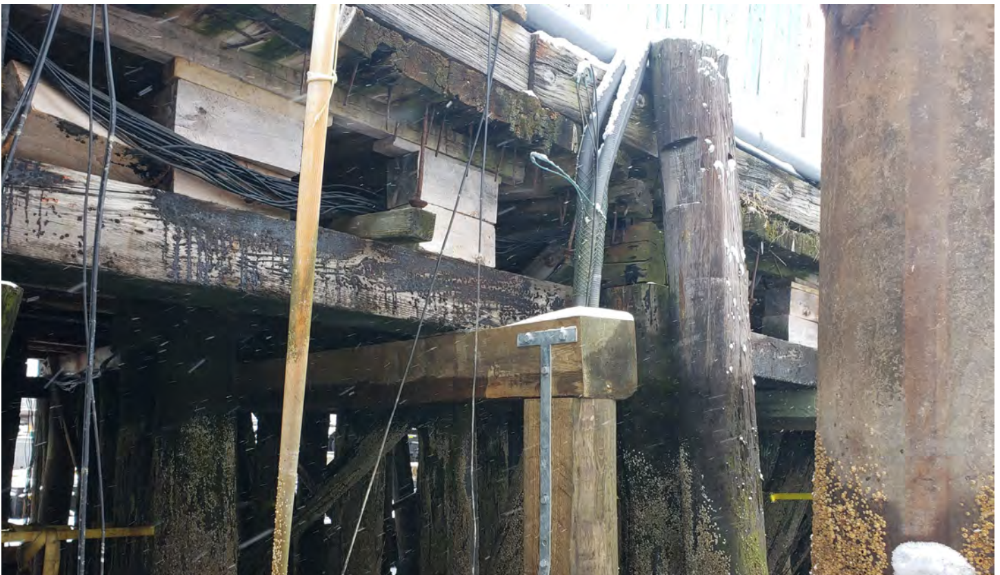
After: The decking is no longer sitting on the power cables and has been raised.
