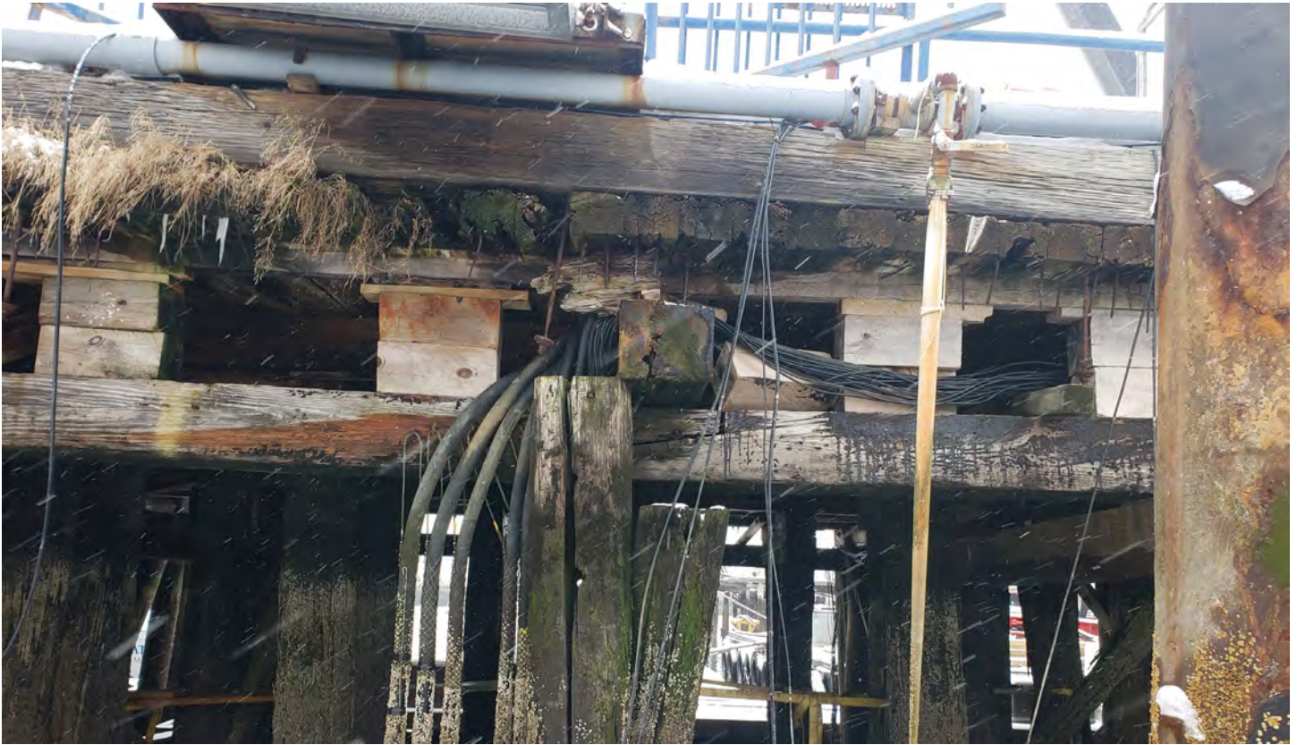
Before: Decking is collapsed onto the power cables below the electrical transformer.
