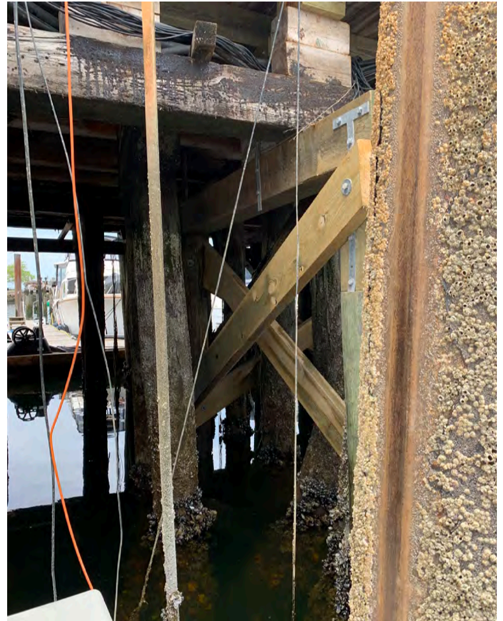
Looking west at recently installed bracing and pile caps on the Project Site.
