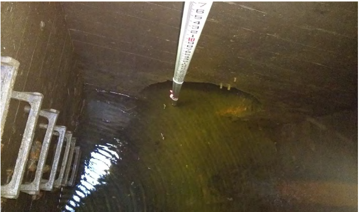
Photo #11: View into the open vault of the 54” tide gate. Vault repair and two new drain lines are proposed.
