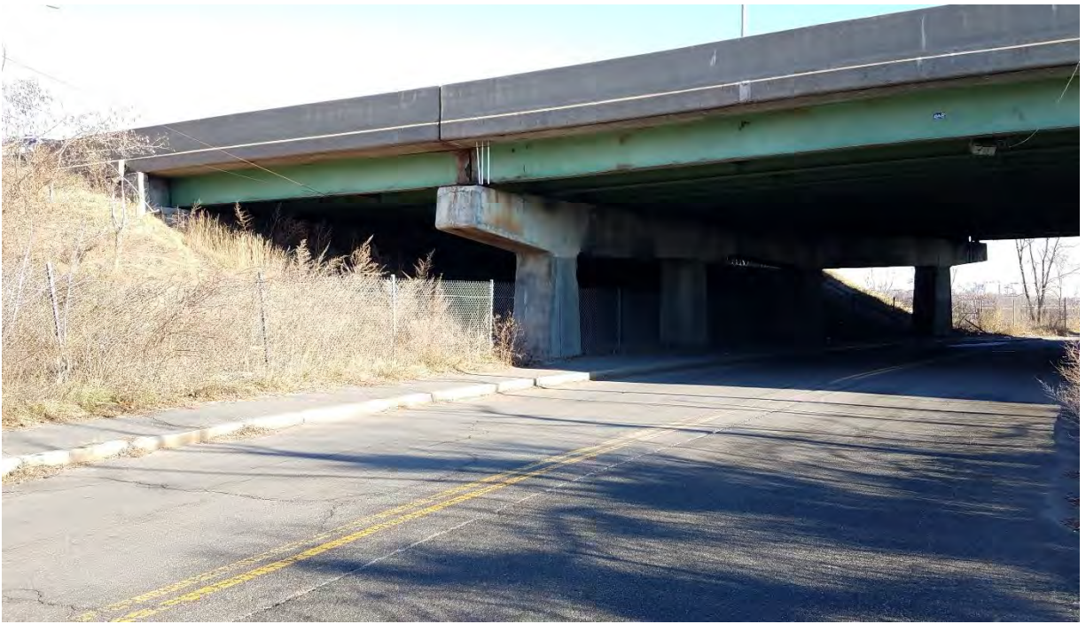
Photo #14: View of the expressway overpass crossing Conley Street. A new roadway cross section is proposed in this area to accommodate the trail and improve connectivity in LSCSF. Facing generally east.
