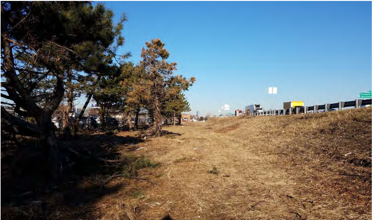
Photo #9: Additional view of conditions along the western embankment of the expressway, in the vicinity of the proposed pathway. Facing north
