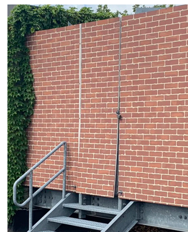
Existing faux brick to be replaced
