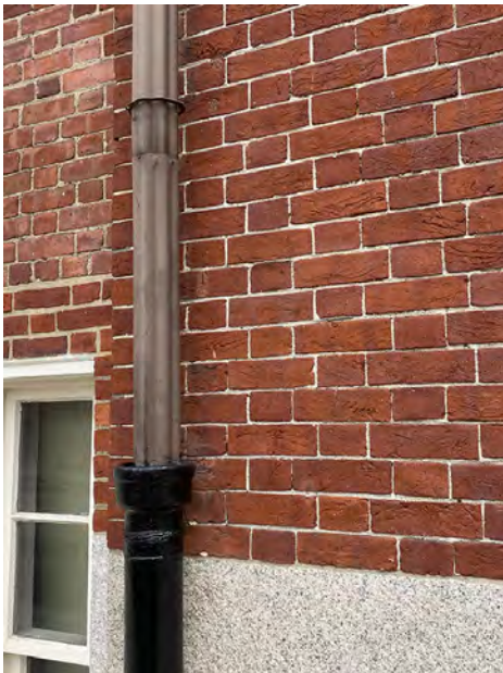
BASE OF PAINTED COPPER DOWNSPOUT AT STREET LEVEL CONNECTION TO PAINTED CAST IRON RAIN LEADER BOOT
