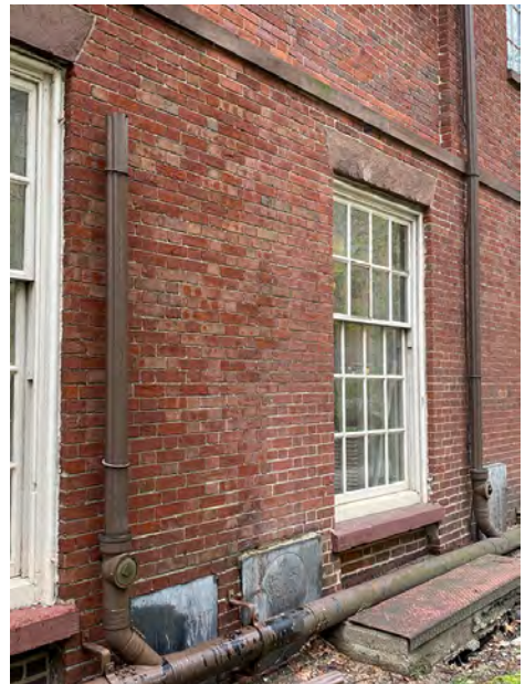
SECTION OF DOWNSPOUT AT GRANARY FACADE RECENTLY DISLODGED DURING WIND STORM
