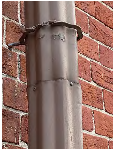
EXISTING BRACKET WITH STEM BROKEN AT CONNECTION TO WALL
