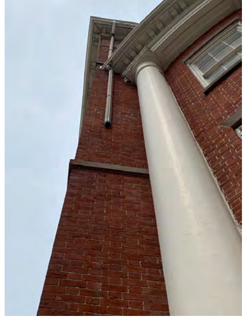
SECTION OF DOWNSPOUT RECENTLY DISLODGED DURING WIND STORM
