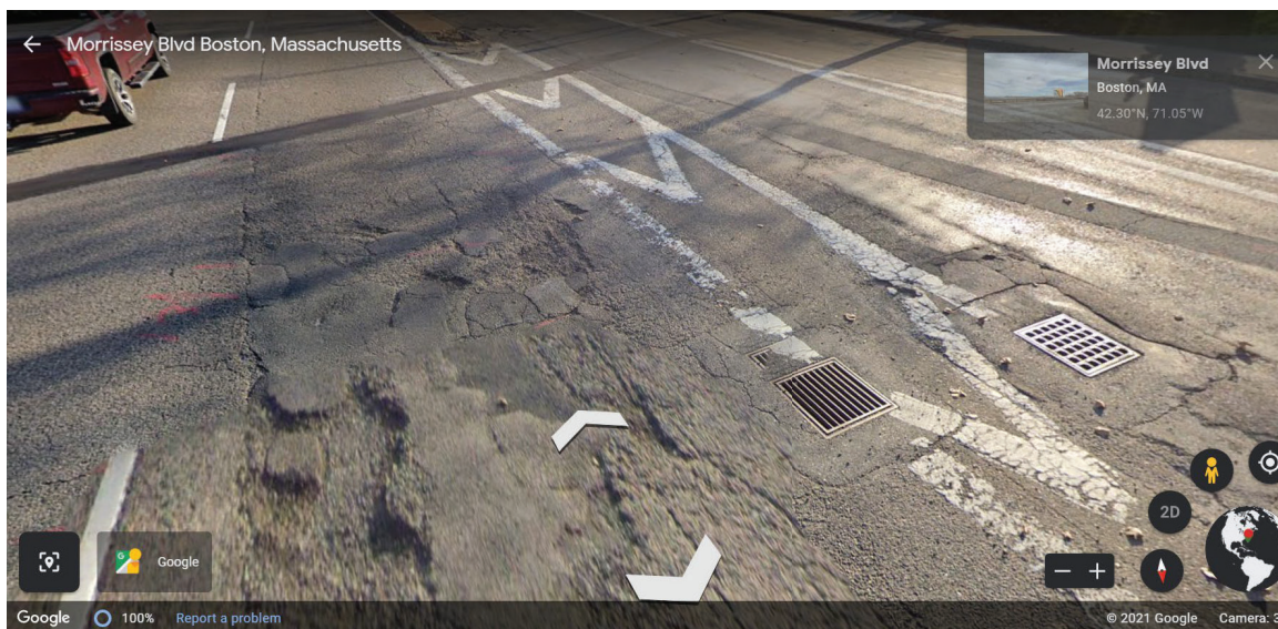
Photo 2. Example of poor road condition and existing catch basins at Morrissey Boulevard.
