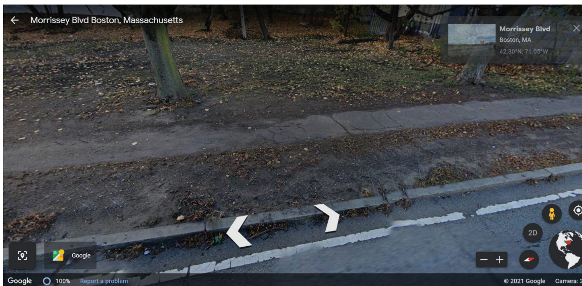
Photo 6. Example of poor sidewalk condition adjacent to Morrissey Boulevard.
