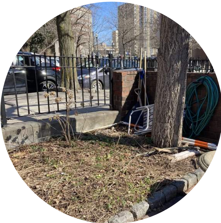
Grade change and existing concrete retaining wall at edge along Charles Street
