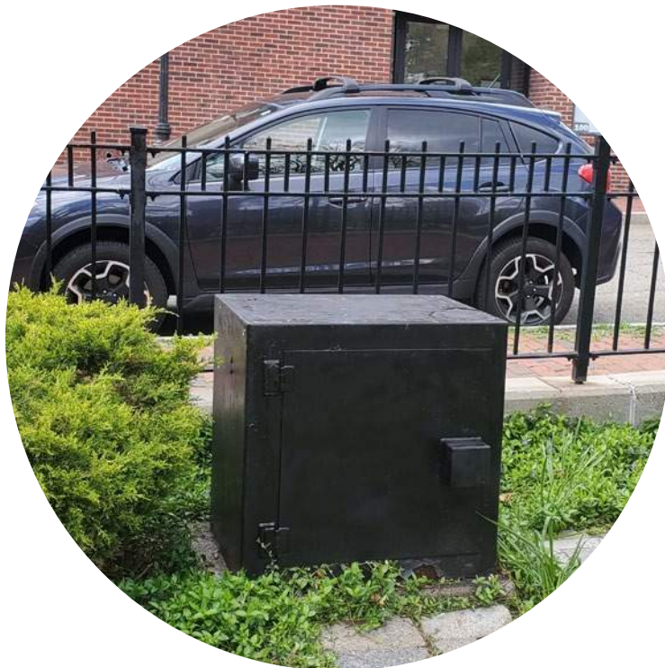
Fountain mechanical equipment box, in need of repair
