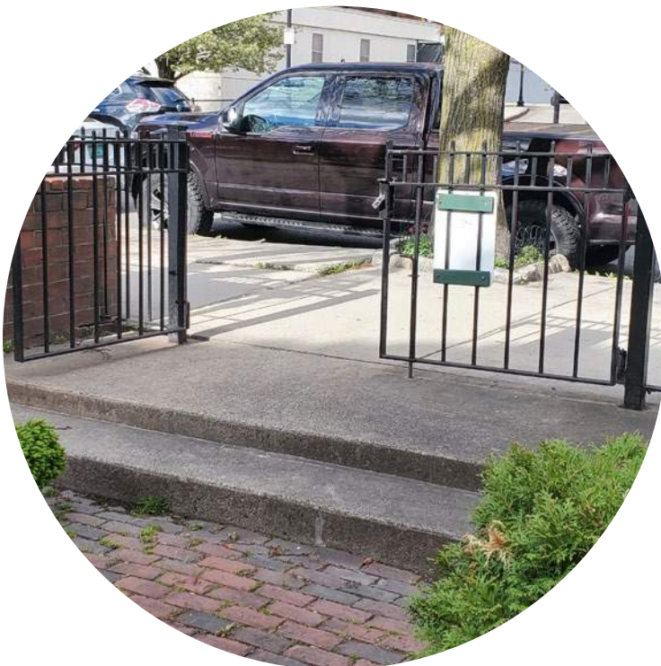
Inaccessible Charles Street entrance
