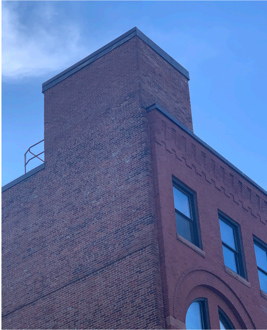
Existing Elevator Machine Room
