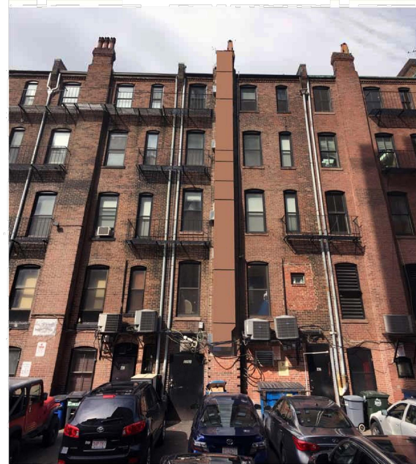
PROPOSED VIEW OF PIATTINI VENT DUCT TO BE PAINTED BRICK COLOR (Benjamin Moore Paint Color/Name: HC- 50 /Brick)
