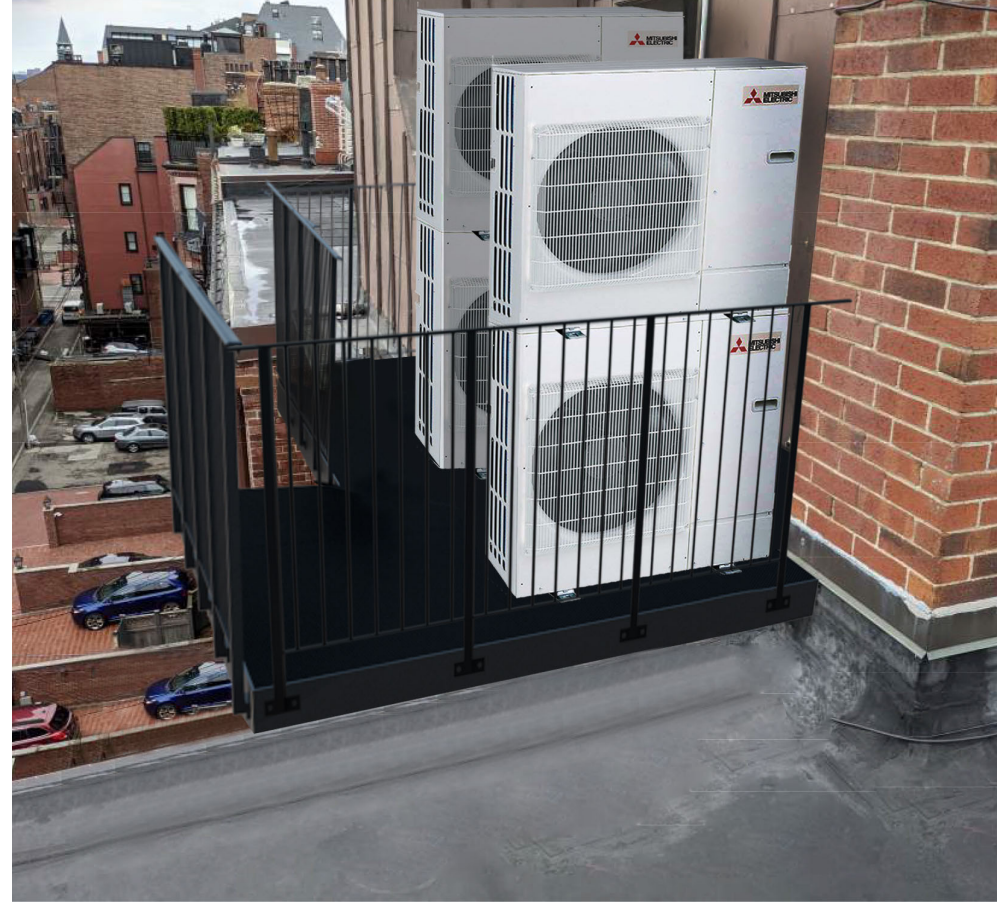
PROPOSED HVAC UNITS WITH GUARD RAILINGS
