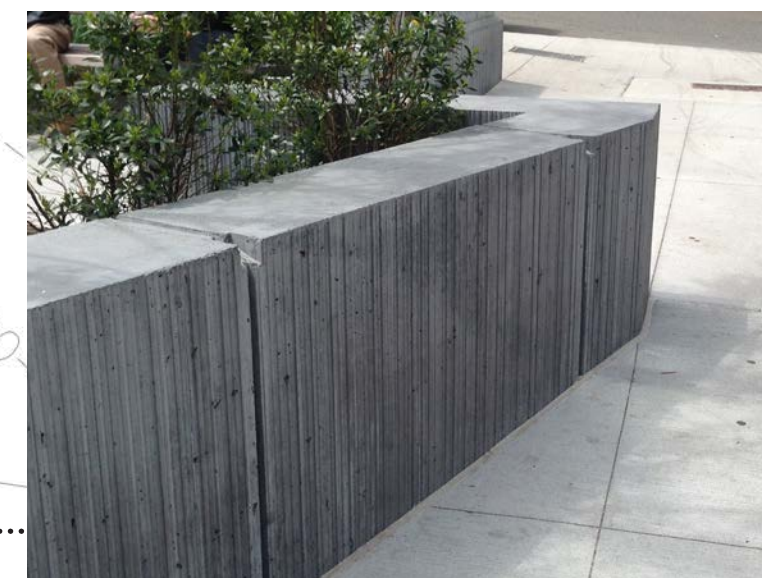
RETAINING WALL Large precast concrete block retaining wall to enclose depressed parking area
