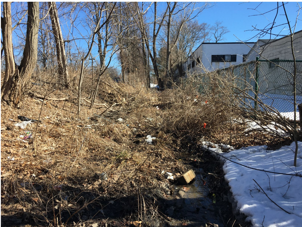
View to East up the Drainage Showing Fence, Various Debris, and Vegetation Overgrowth
