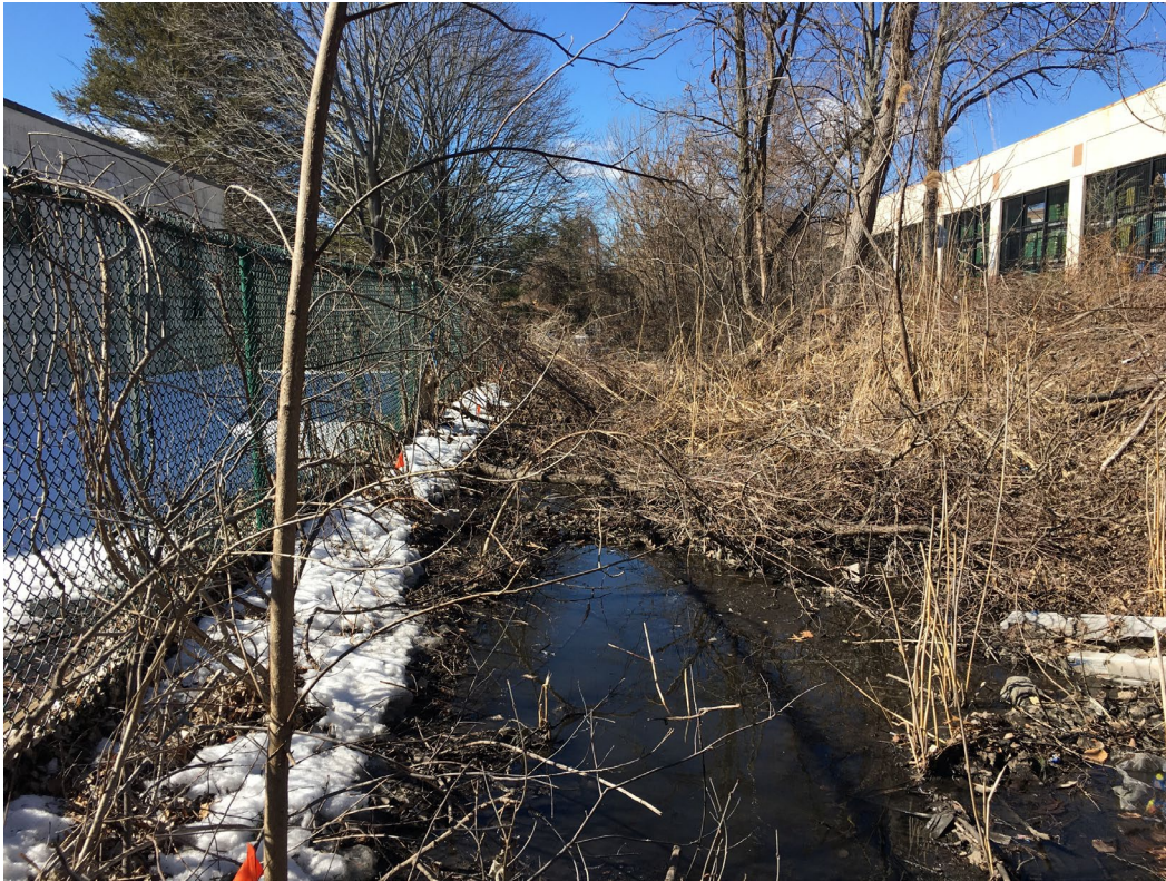
View to West Along Drainage Showing Home Depot Fence and Vegetation Overgrowth
