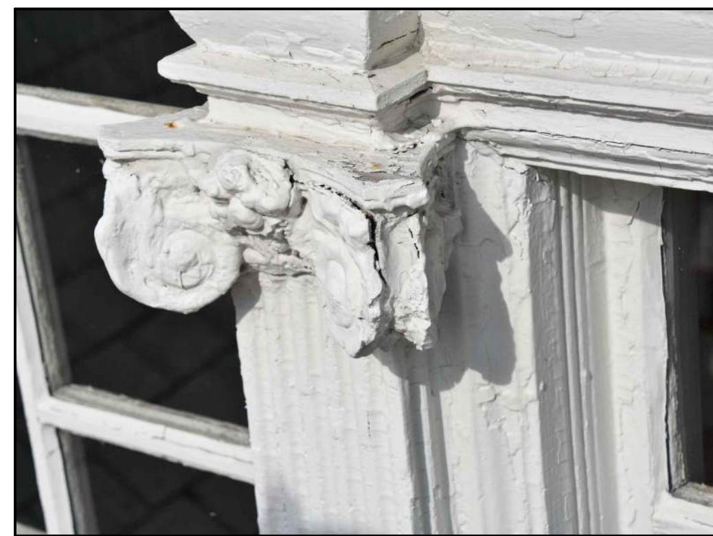
8 DAMAGED CAPITAL AT DORMER
