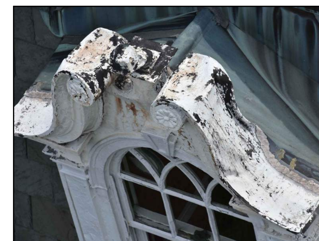
4 DAMAGE AT ROOF DORMER
