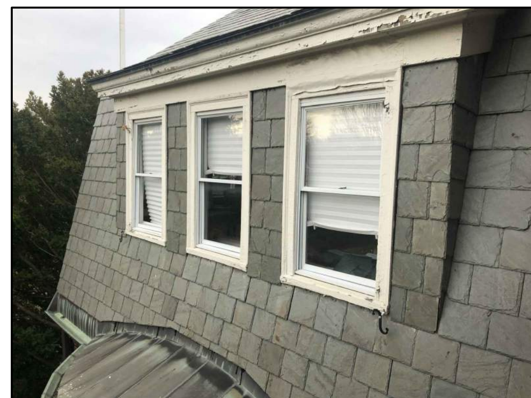
9 WINDOWS TO BE REPLACED
