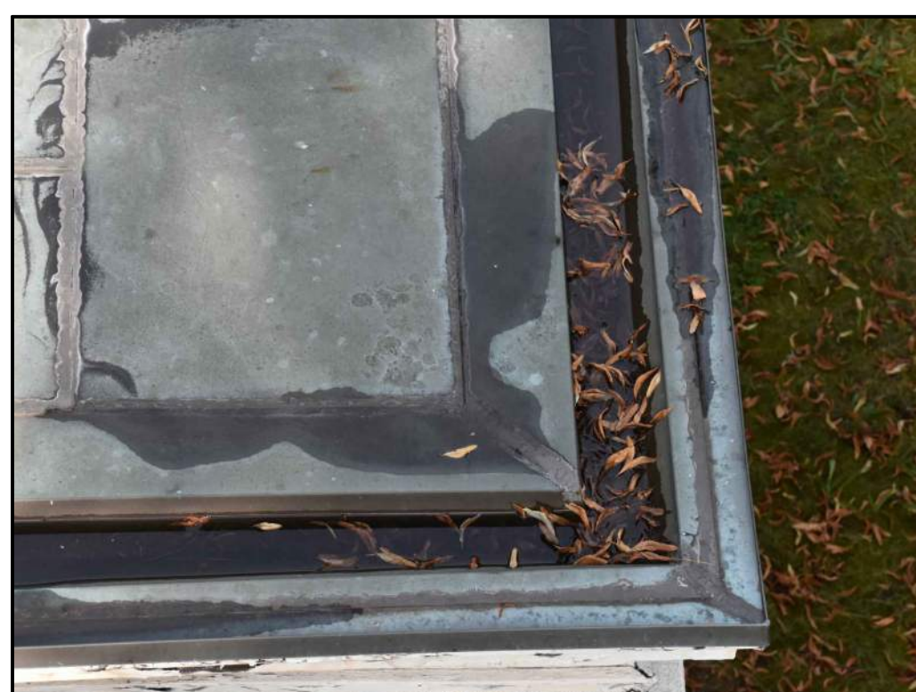
18 SUNROOM ROOF - GUTTER
