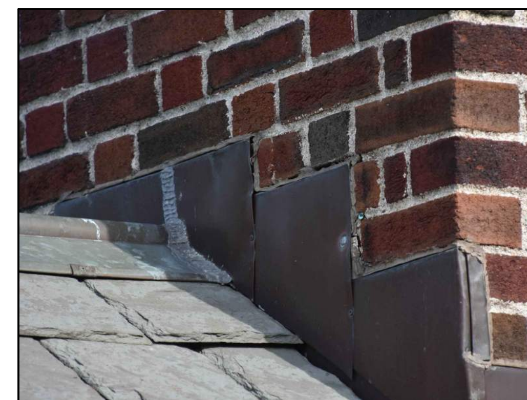
8 FAILED SEALANT AT FLASHING
