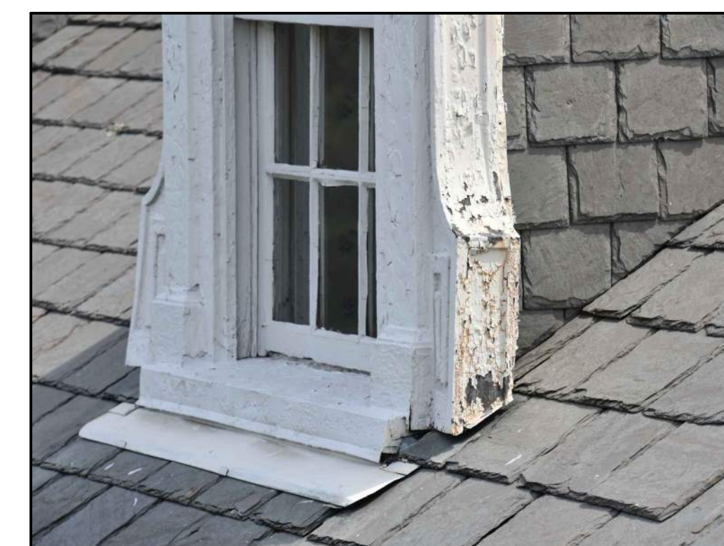
2 DAMAGE AT ROOF DORMER - WEST
