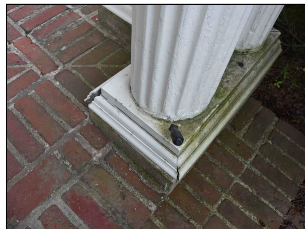
13 DETERIORATING COLUMN BASES
