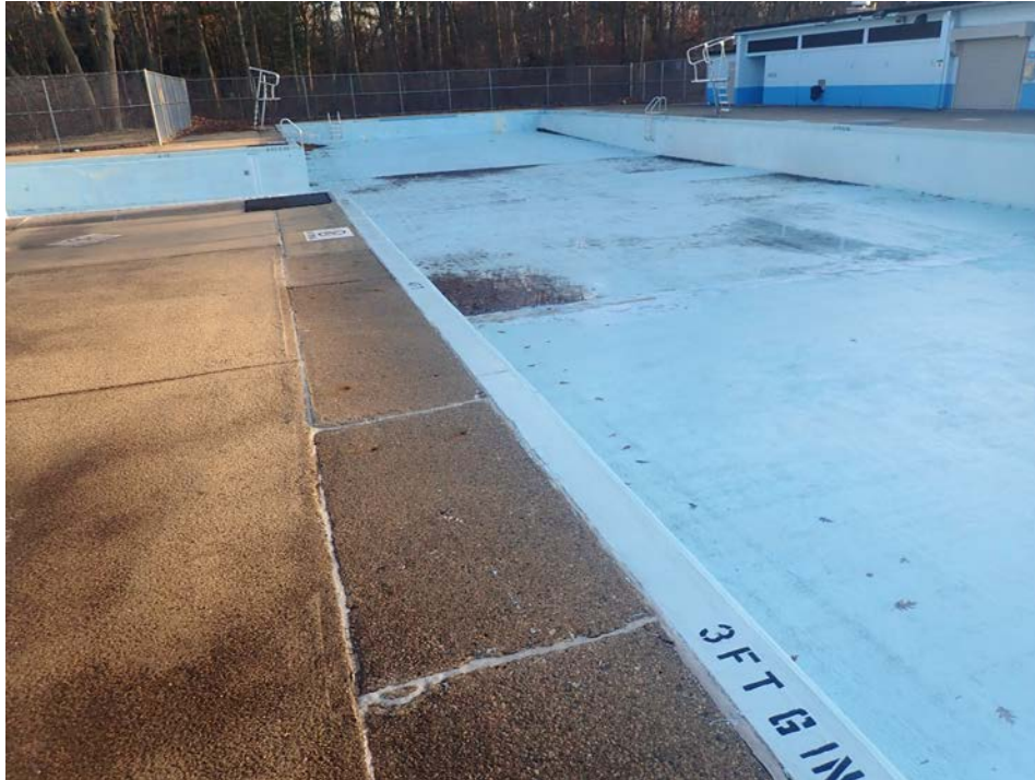
Photo 2 – View of the concrete pool deck and the blue pool interior shell as viewed from the northwest.
