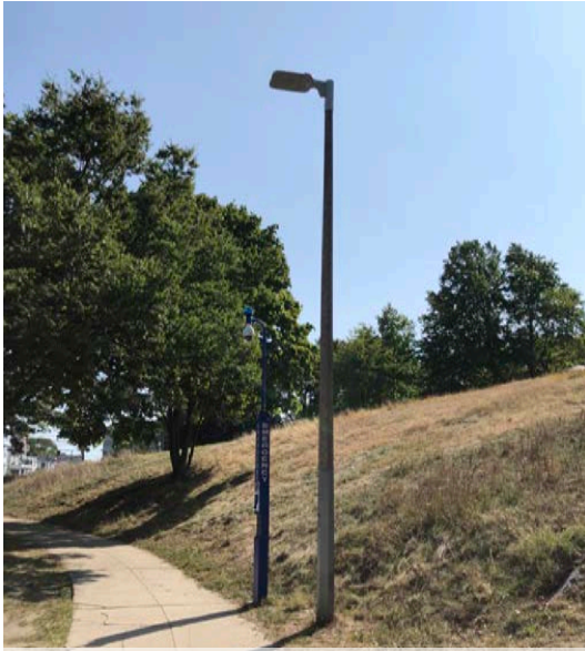
LIGHTING FIXTURE AND EMERGENCY TELEPHONE
