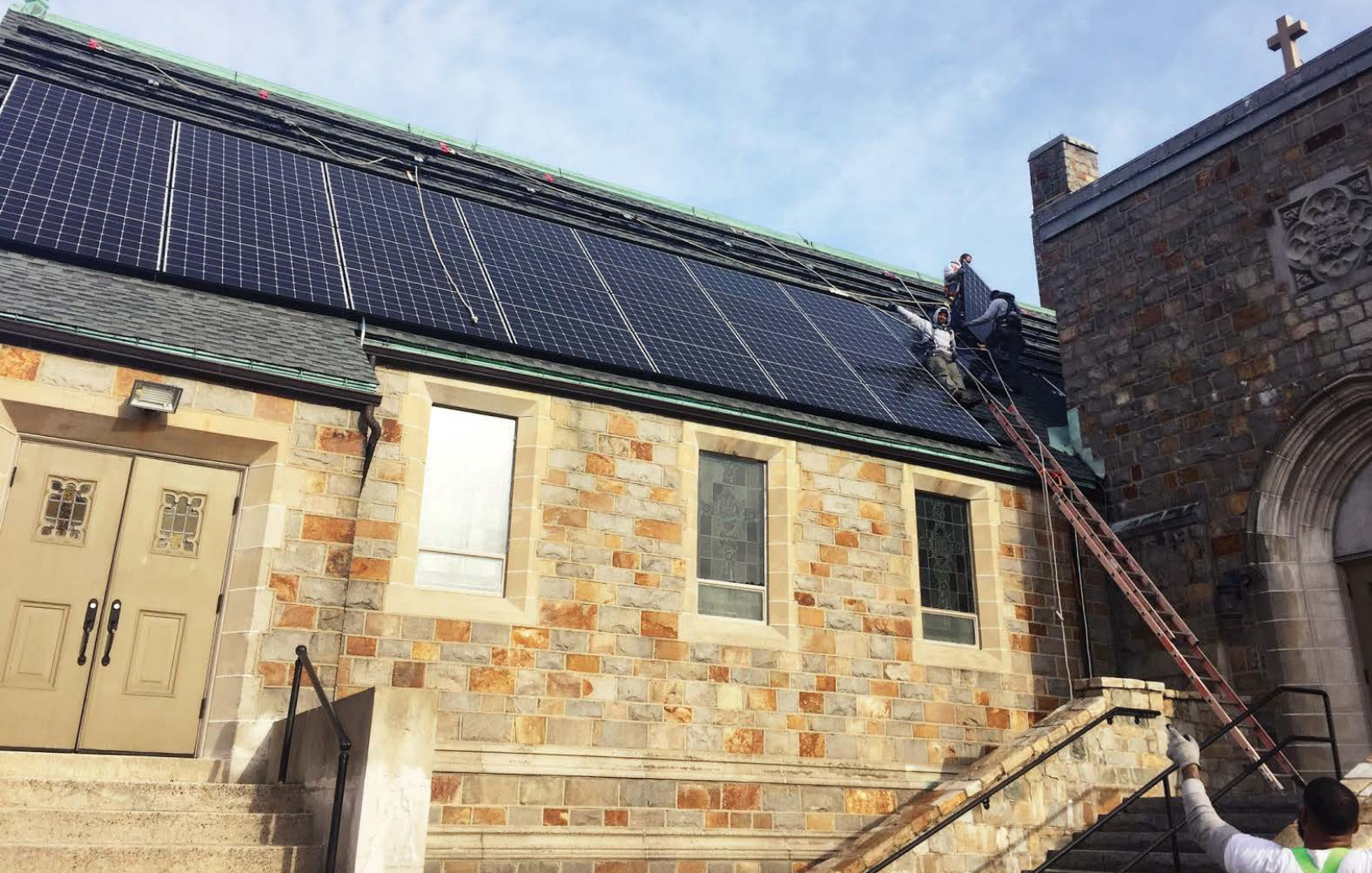
Solar Installation on Bethel AME Church in Jamaica Plain. Photo credit: Resonant Energy
