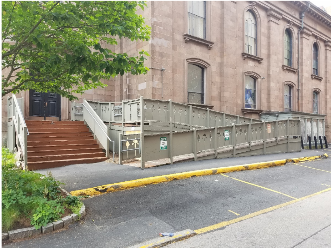
North elevation of stair and ramp with basement enclosure in the back
