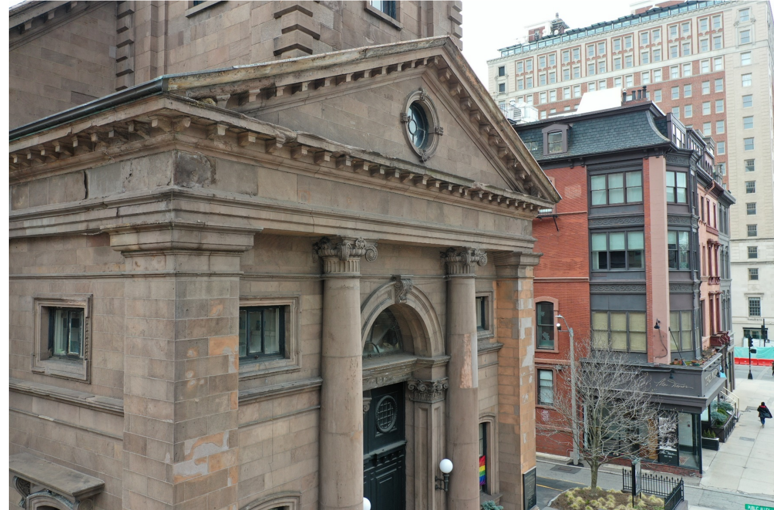
View of portico projecting cornice with multiple spalls and large crack
