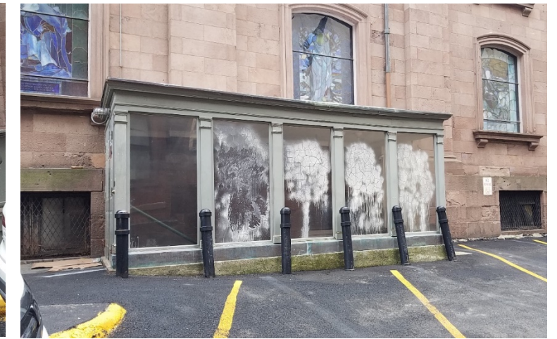
Existing basement stair enclosure wood structure is deteriorating and plexi-glass window film is cracking
