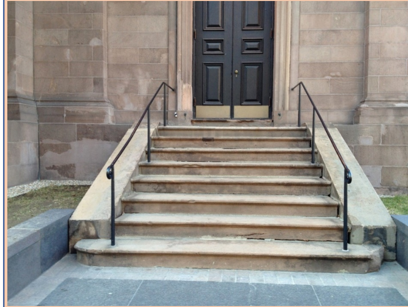
Photograph of existing south stairs before removal. Note step at door and shallow landing
