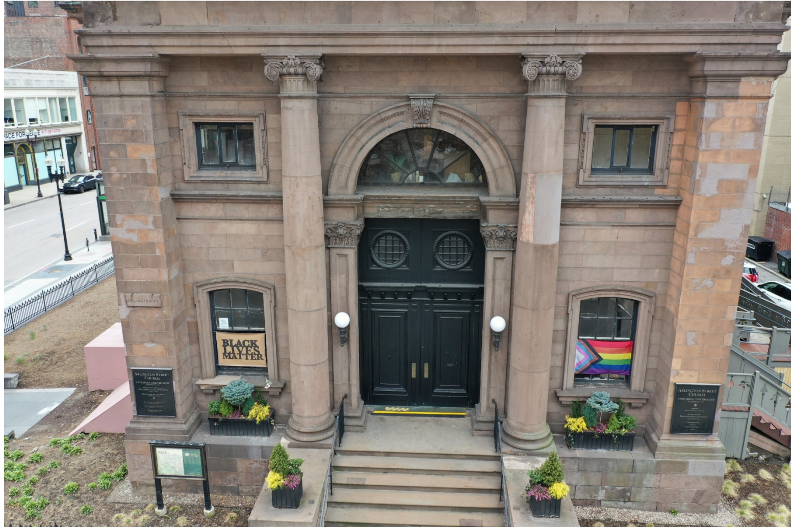
View of east façade with stains and failing composite repair mortar patches
