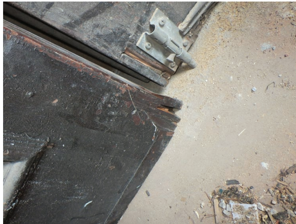
SPLINTERING AT DOOR CORNERS
