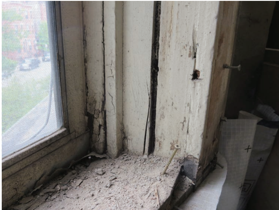
WINDOW 'F' - SILL AND FRAME DAMAGE
