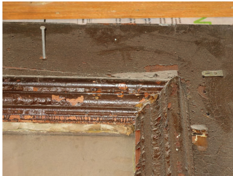
MOULDING IS SEPERATING FROM THE DOOR
