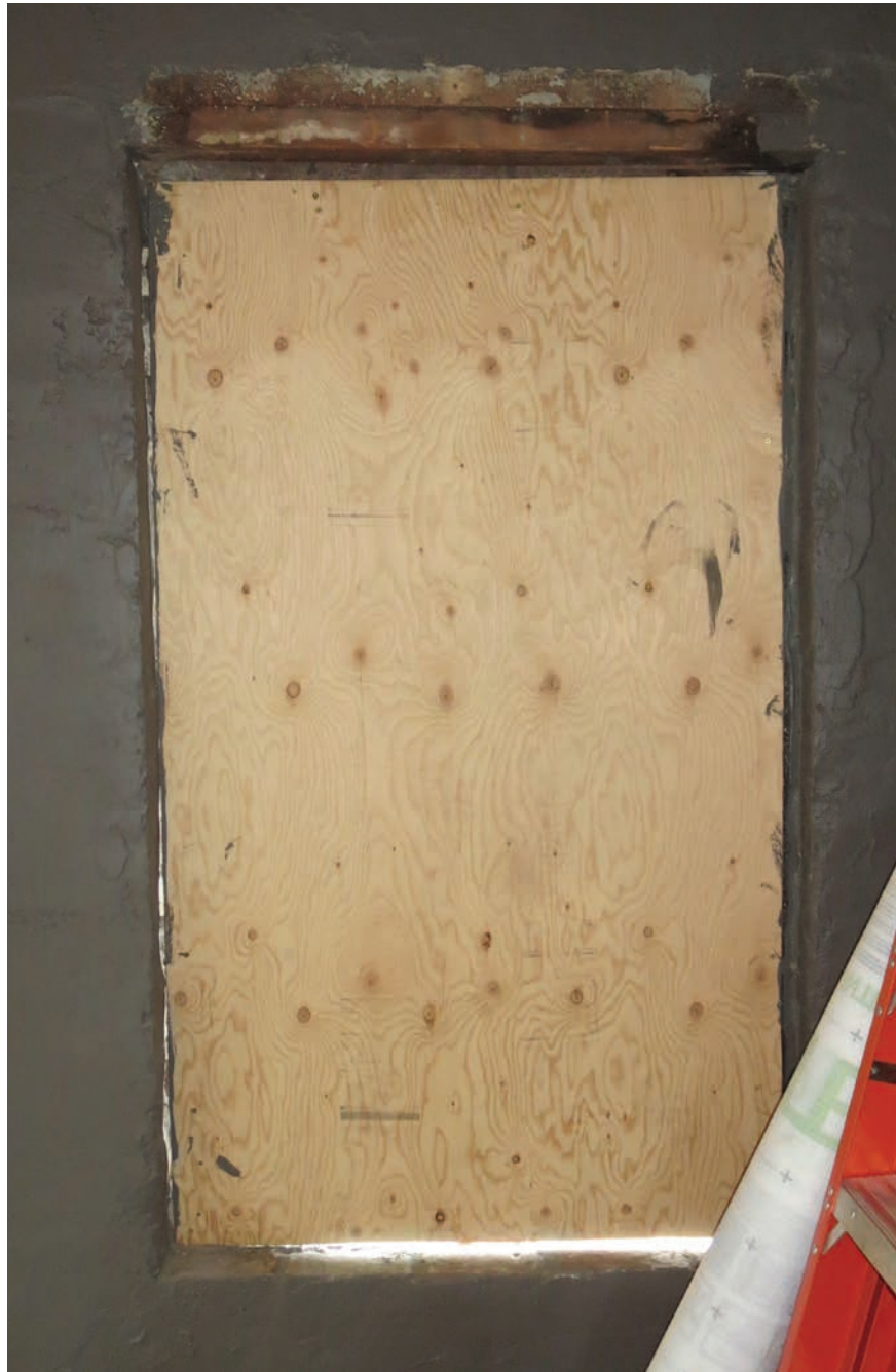
WINDOW 'A' - FOURTH FLOOR (MISSING)
