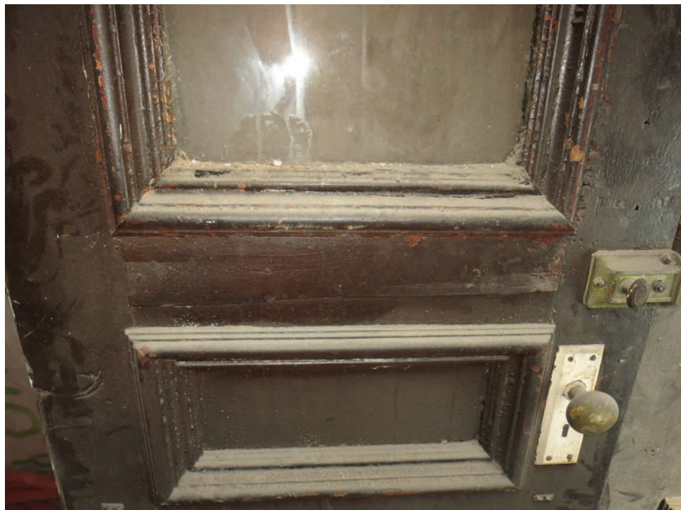
CRACKING AT RAIL
