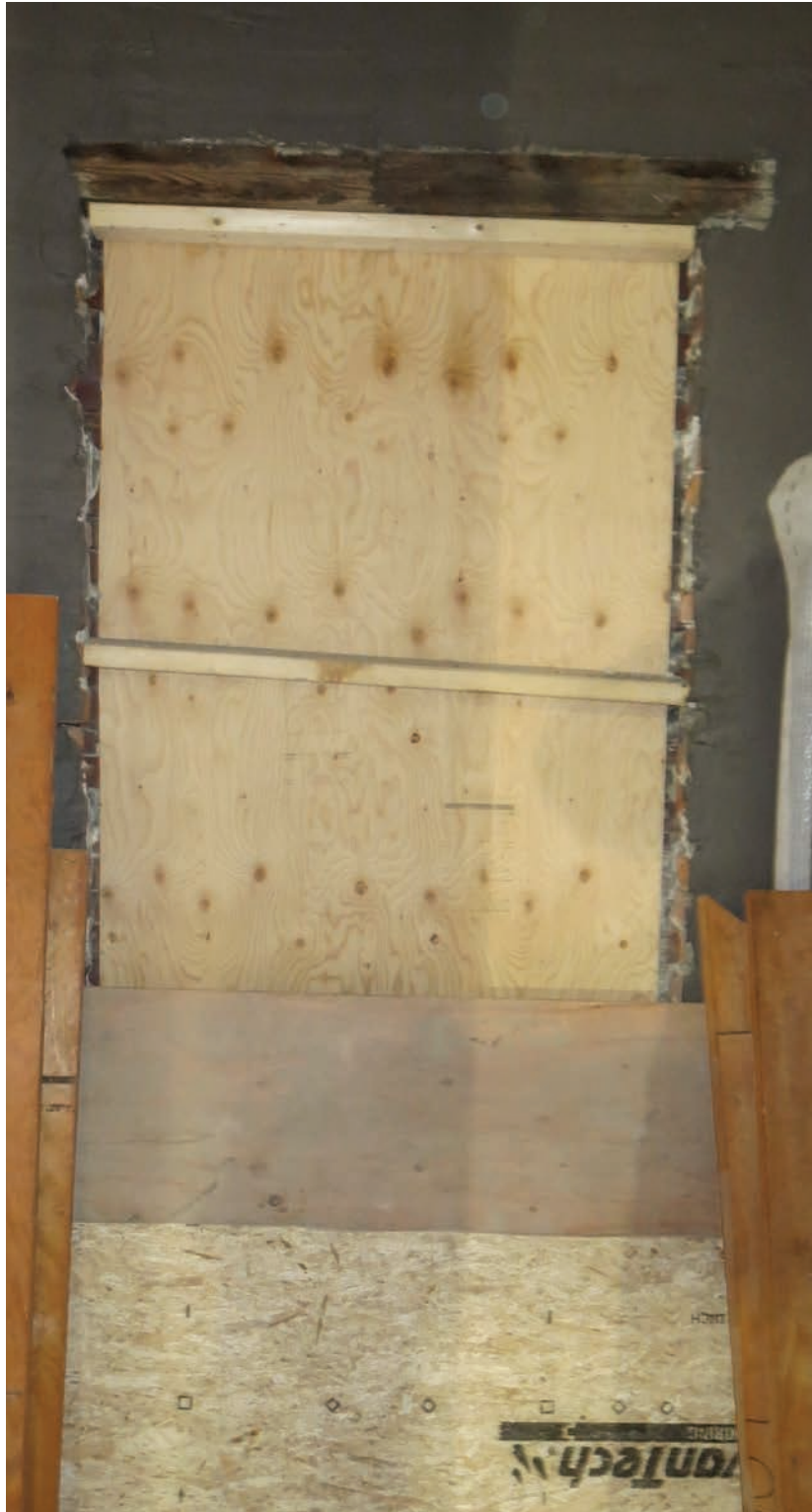
WINDOW 'D' - FOURTH FLOOR (MISSING)
