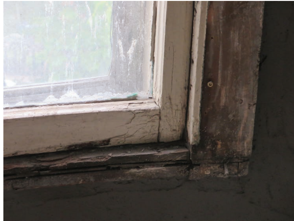
WINDOW 'C' - FRAME AND SASH DAMAGE
