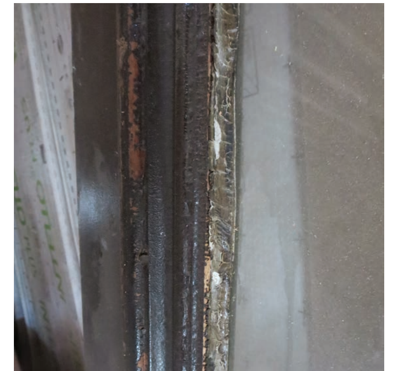
PUTTY GLAZING CRACKING
