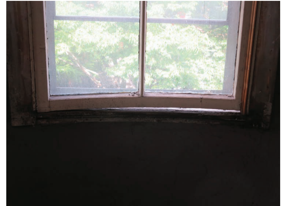
WINDOW 'B' - FRAME AND SASH DAMAGE MISSING WINDOW STOP
