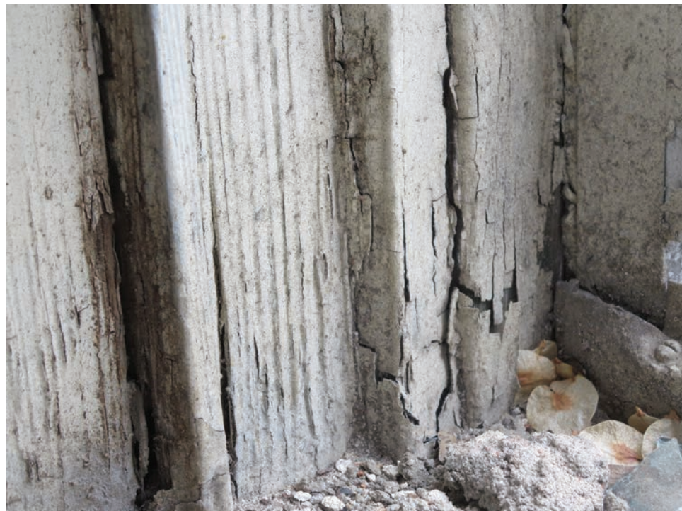
WINDOW 'E' - FRAME DAMAGE
