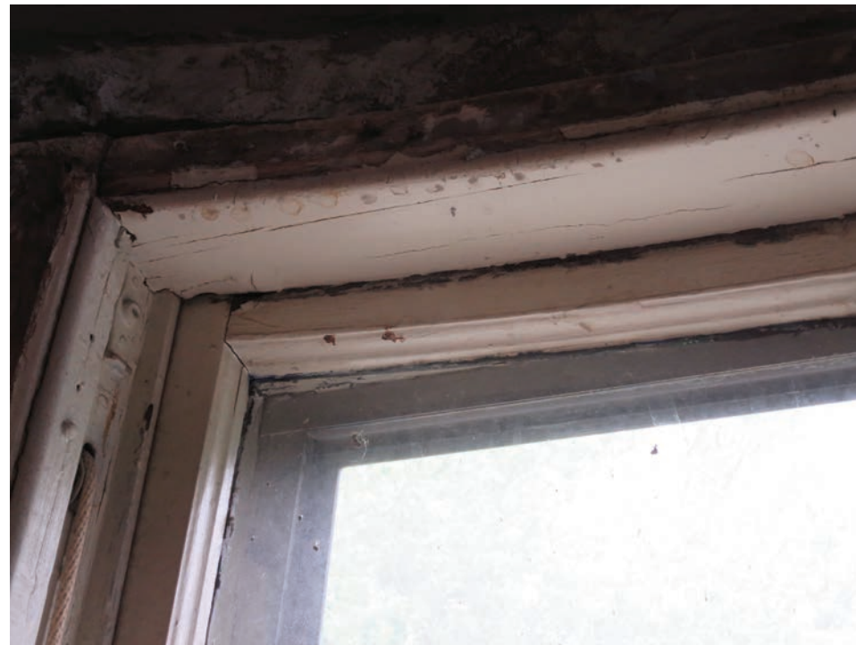
WINDOW 'E' - FRAME AND SASH DAMAGE
