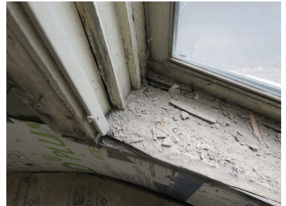
WINDOW 'F' - SILL AND FRAME DAMAGE
