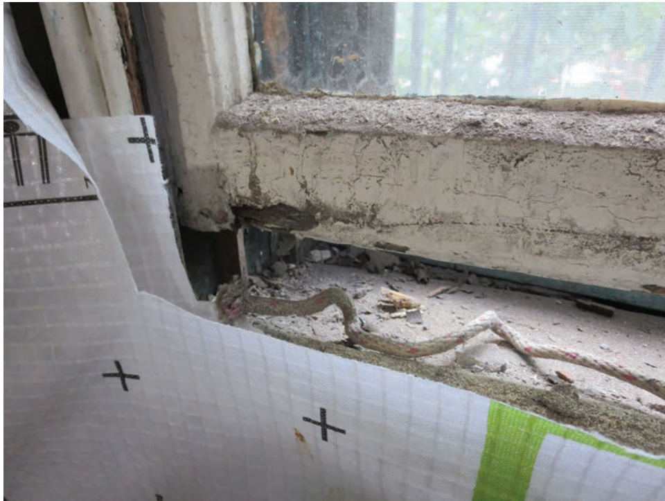
WINDOW 'H' - SASH DAMAGE COUNTER-WEIGHT NEEDS REPLACED
