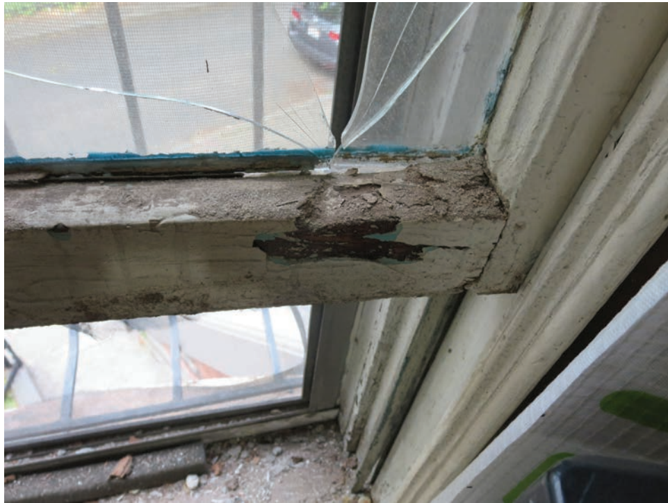
WINDOW 'G' - SASH DAMAGE BROKEN GLASS PANE
