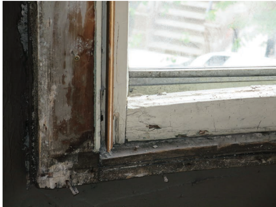
WINDOW 'C' - FRAME AND SASH DAMAGE BROKEN GLASS PANE
