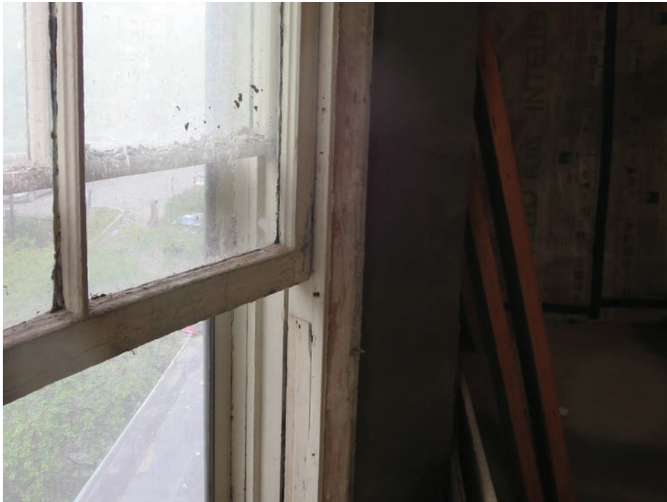
WINDOW 'F' - MISSING WINDOW STOP
