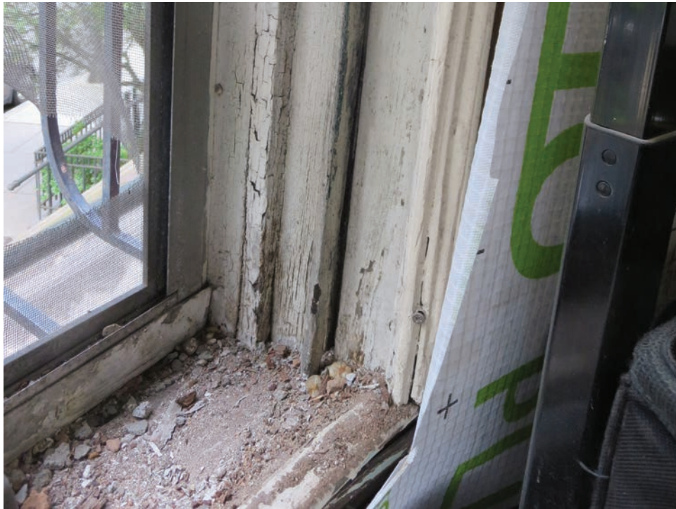
WINDOW 'G' - SILL AND FRAME DAMAGE
