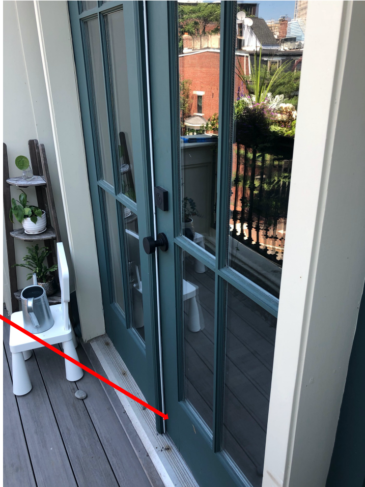
Exterior deterioration – water leaking and door swelling
