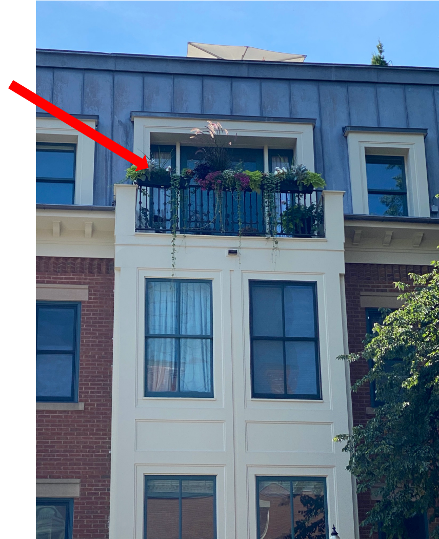
Failing Doors and Side lites – Structure built in 1997
