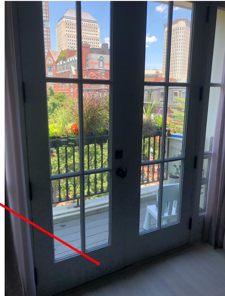
Interior Deterioration – water leaking and door swelling
