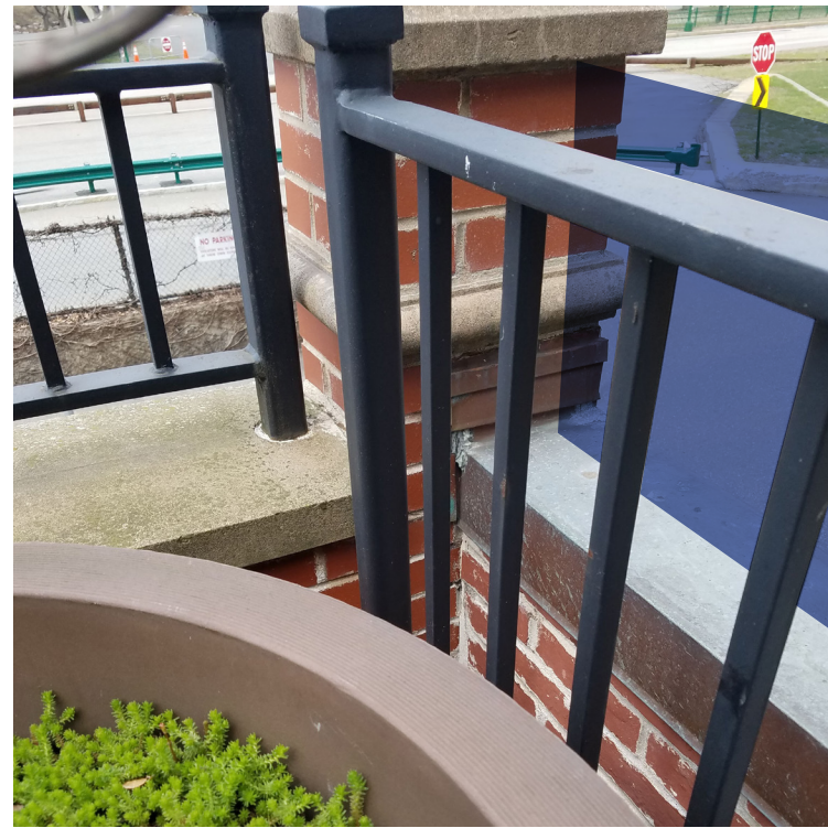
Far Left: Existing railing condition, the gap between railing and parapet is lost deck space and debris trap. Proposed railing location is highlighted in dark blue.
