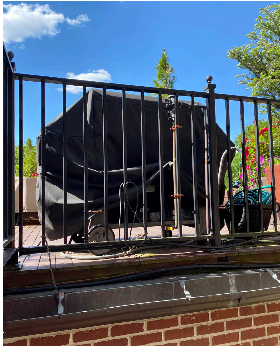
South Elevation Detail of existing exposed hard pipe grill and irrigation connections
