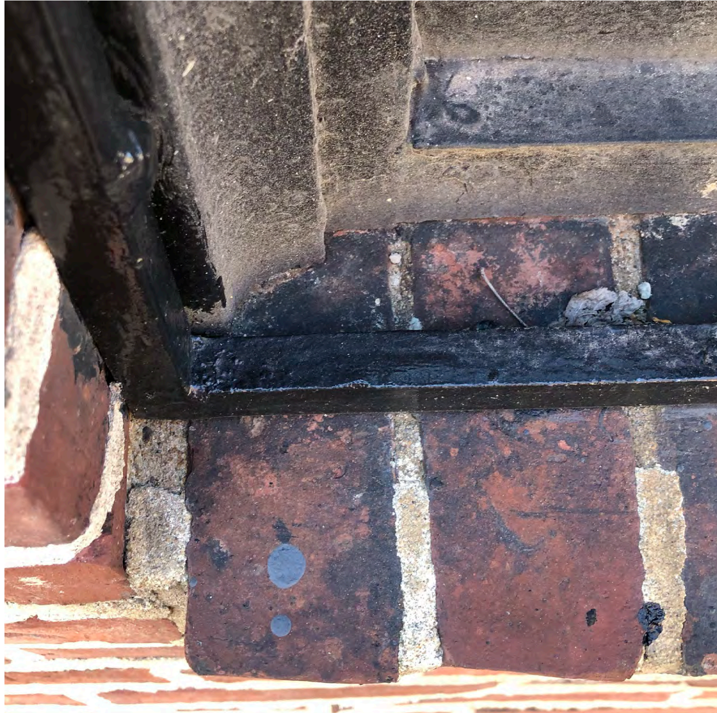
WINDOW C LEFT SIDE SILL
