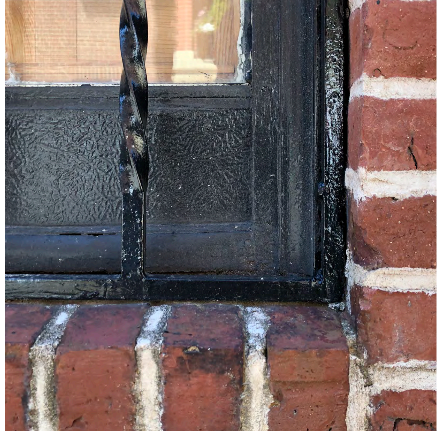
WINDOW A RIGHT SIDE SILL
