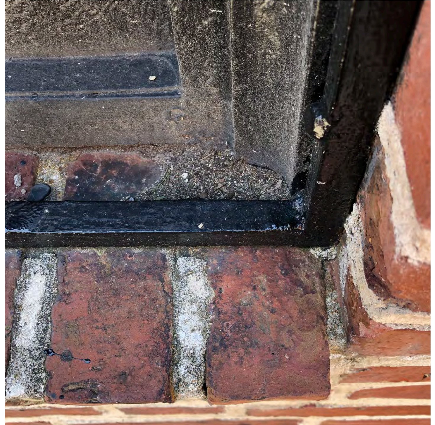
WINDOW A RIGHT SIDE SILL
