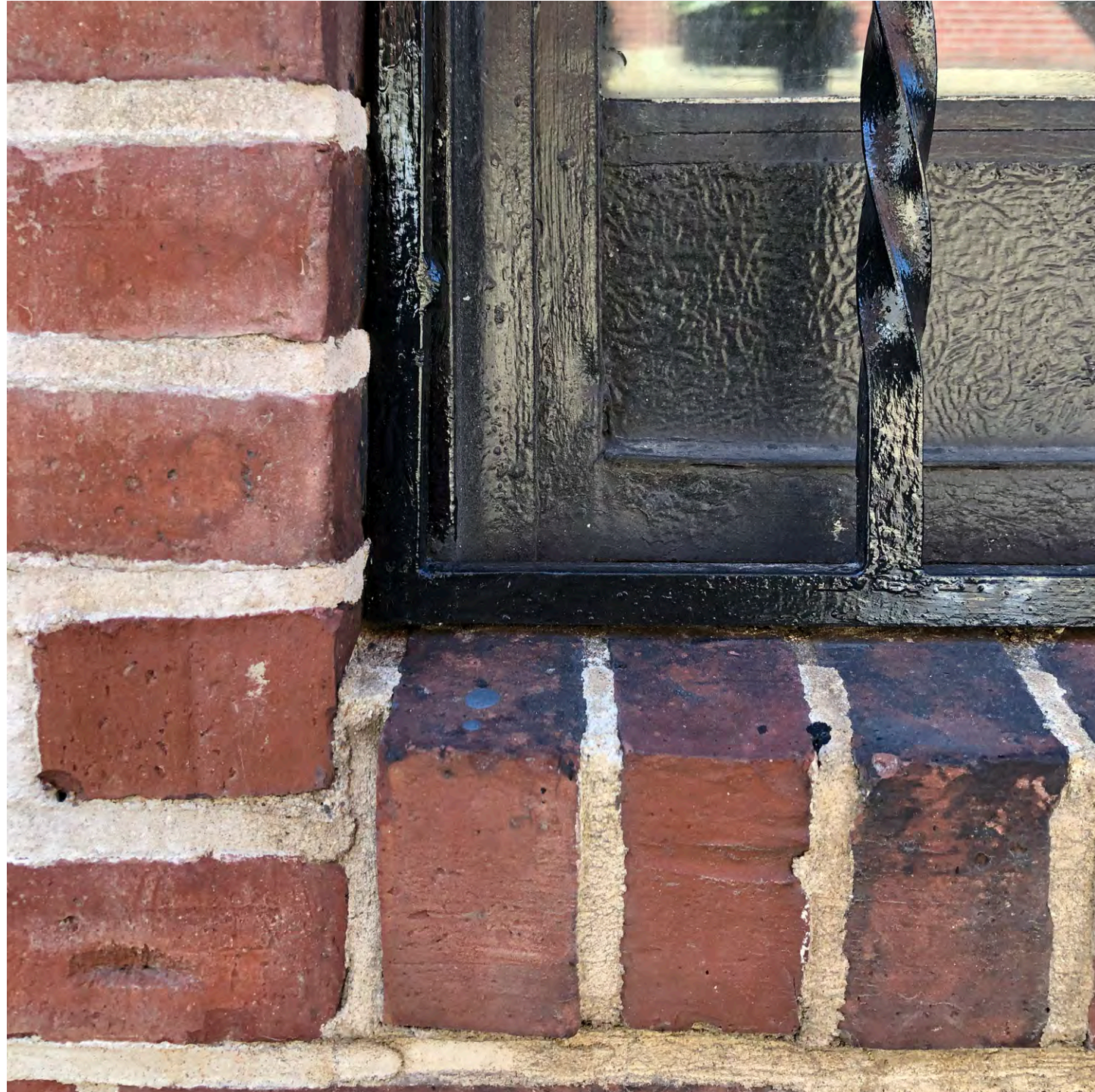
WINDOW C LEFT SIDE SILL
