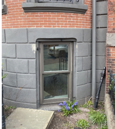
Block to be repainted grey from gutter to entry
