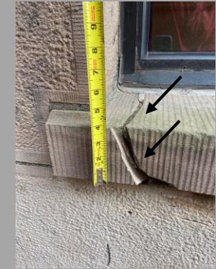
PHOTO 3 – EXAMPLE OF CRACKED SILL STONE (ARROW).
