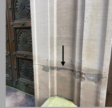
PHOTO 11 – EXAMPLE OF MIS-MATCH PREVIOUS MORTAR REPAIR (ARROW) NEAR MAIN ENTRY (AT LEFT).
