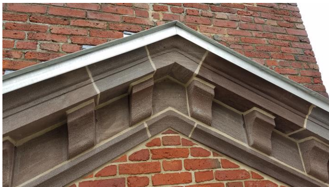
PHOTO 14 – NATURAL STONE REPLACEMENT PIECES INSTALLED AT HARVARD HALL CORNICE, JOINT PATTERNING MATCHES ORIGINAL.
