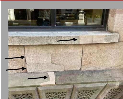
PHOTO 9 – EXAMPLE OF MIS-MATCH PREVIOUS REPAIRS (ARROWS).
