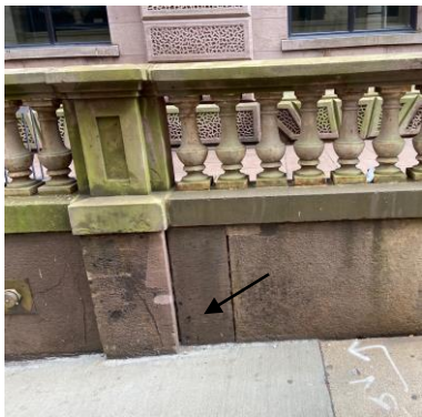
PHOTO 17 – OVERVIEW OF TERRACE WALL, WITH CRACKED STONE (ARROW) NEAR GRADE.
