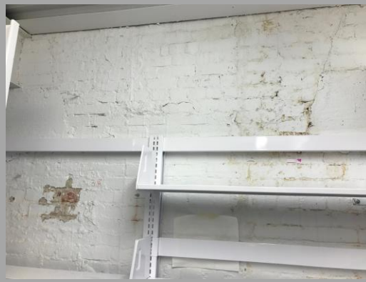
PHOTO 6 – WATER DAMAGE AT INTERIOR (WHERE SENSITIVE COLLECTIONS ARE STORED) FROM THIRD-FLOOR GUTTER.
