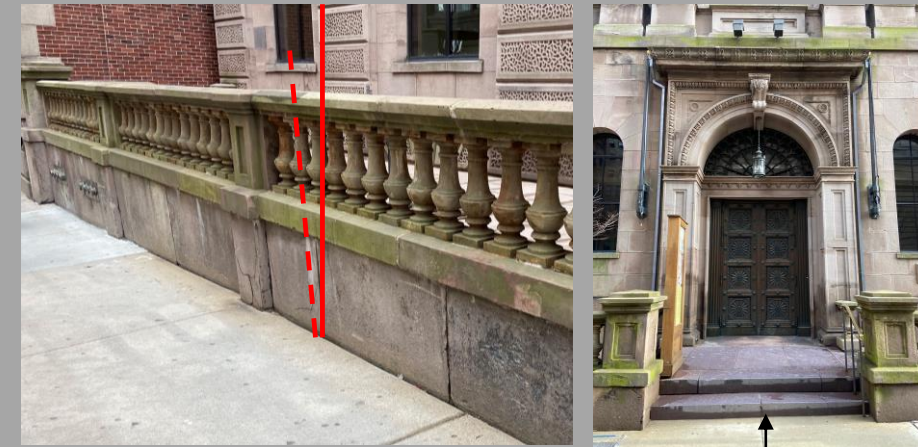
PHOTO 16 – LEFT: ORIGINAL FREE-STANDING WALL AT INFILLED TERRACE IS ROTATED (DOTTED RED LINE RELATIVE TO SOLID RED LINE) DUE TO LATERAL PRESSURES FROM INFILLING THE LIGHTWELL. RIGHT: EXISTING LOCATION OF STAIRS.
