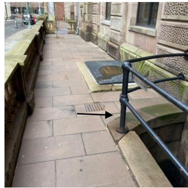
PHOTO 19 – NON CODE-COMPLIANT RAILING (ARROW).
