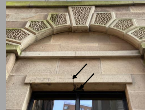
PHOTO 2 – EXAMPLE OF CRACKED AND SPALLED SPANNING STONE (ARROWS).
