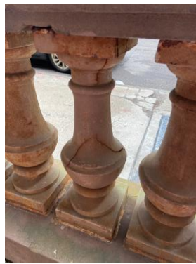
PHOTO 18 – VIEW OF CORRODED AND CRACKED BALUSTRADE.
