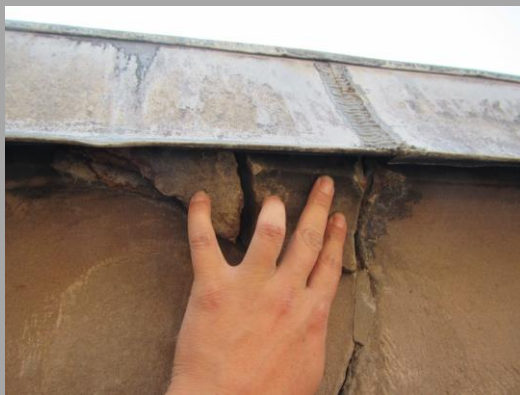
PHOTO 5 – EXAMPLE OF SPALLED STONE BELOW THIRD-FLOOR GUTTER.
