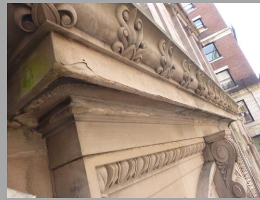
PHOTO 7 – ERODED STONE BELOW UNPROTECTED LEDGE ABOVE MAIN ENTRY..
