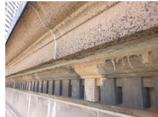
PHOTO 22 – EXAMPLES OF HEAVILY STAINED CAST STONE AT UNDERSIDE OF PROJECTING LEDGES AND DENTILS.
