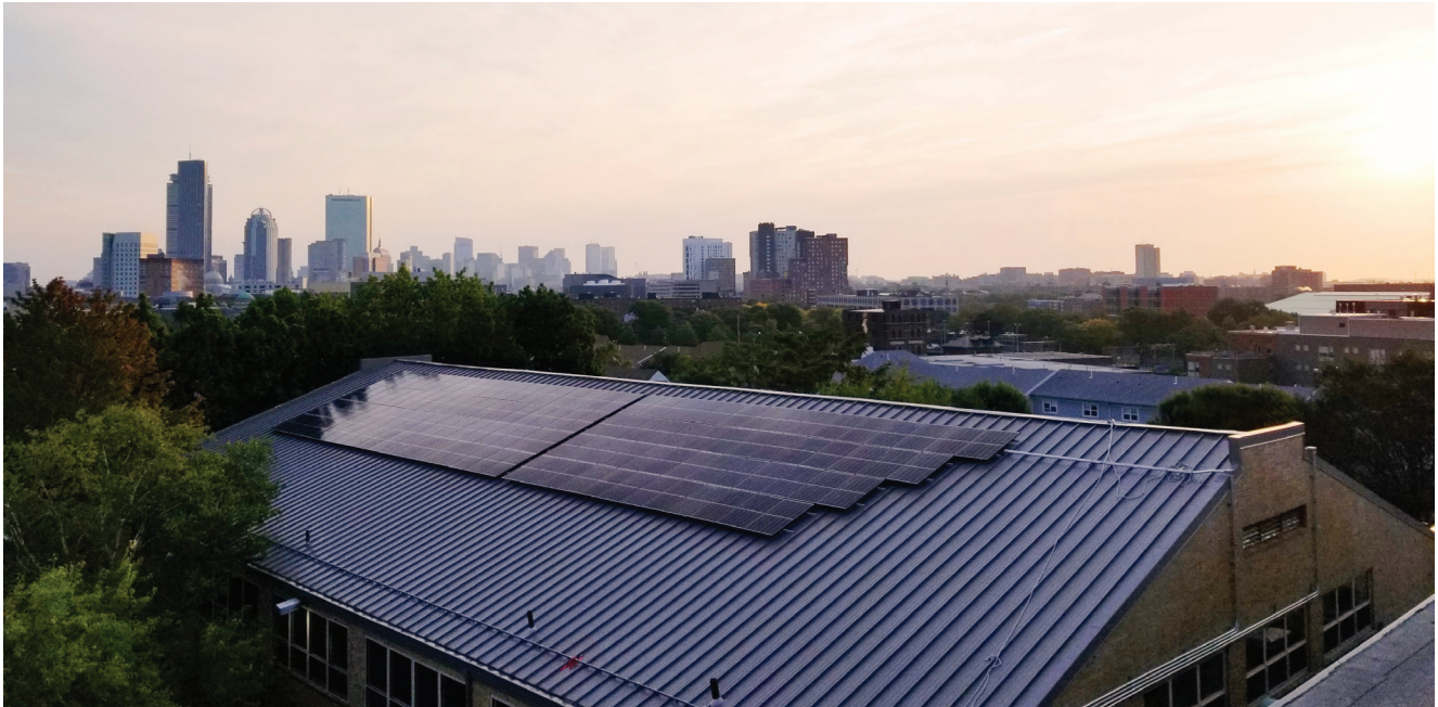
The City of Boston has installed solar panels on the roof of the Tobin Community Center.
