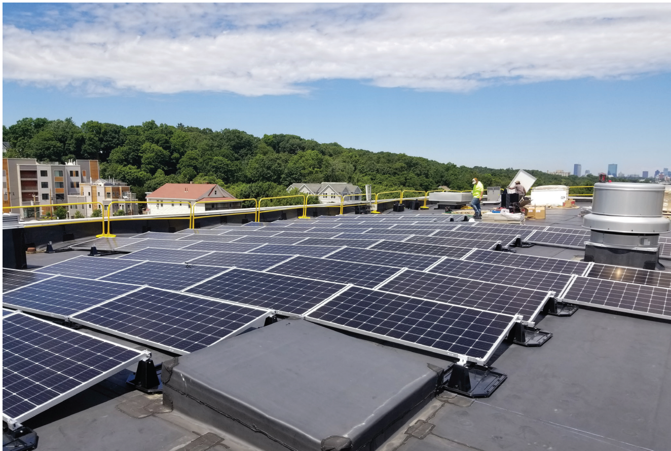
The City of Boston has installed solar panels on the roof of the Roslindale Community Center through the Renew Boston Trust program.
